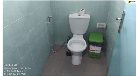
Figure 11 - Missing Toilet Seat Cover
