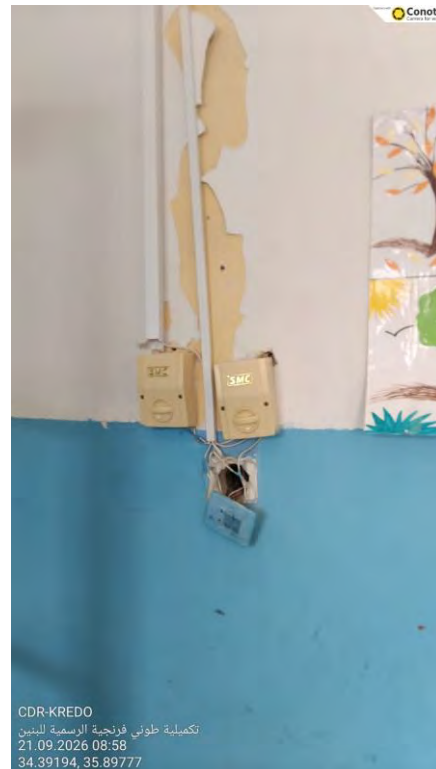
Figure 18 - Damaged Electrical Switch
