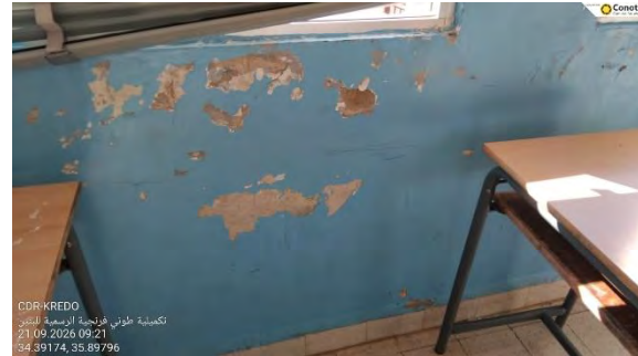
Figure 13 - Damaged Wall Paint
