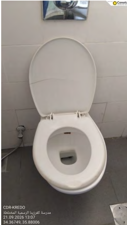
Figure 8 - Broken Toilet Seat Cover
