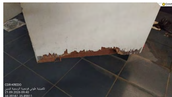
Figure 8 - Damaged Toilet Door
