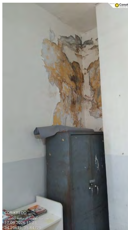
Figure 11 - Humidity in Wall
