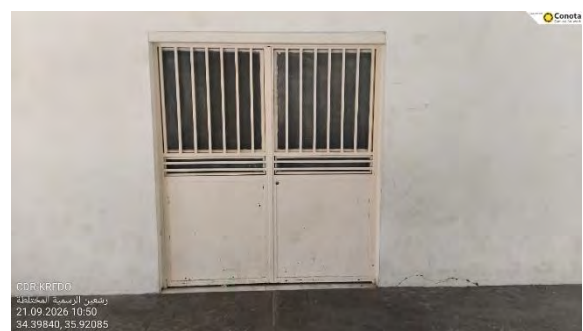
Figure 7 - Damaged Steel Door Paint
