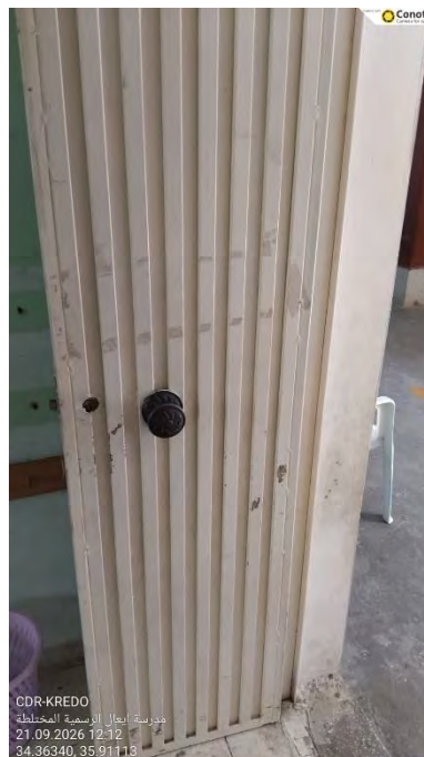
Figure 12 - Damaged Steel Door Paint
