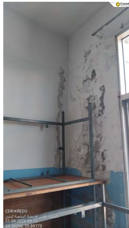
Figure 15 - Humidity in Wall
