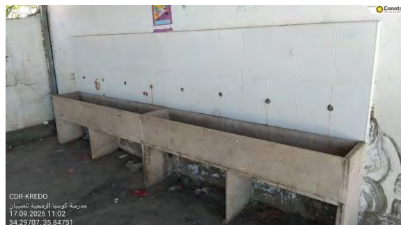
Figure 15 - Missing Drinking Taps
