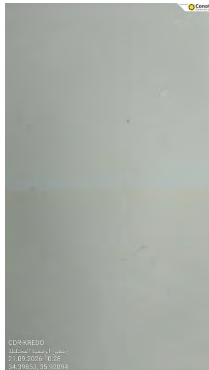
Figure 19 - Crack in Wall
