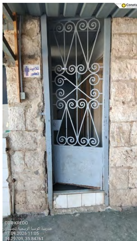
Figure 20 - Damaged Steel Door Paint
