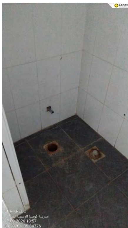
Figure 8 - Missing Toilet Seat
