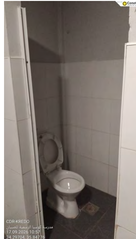
Figure 9 - Missing Aluminum Door
