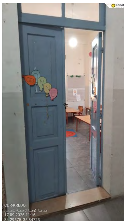
Figure 13 - Damaged Door Paint
