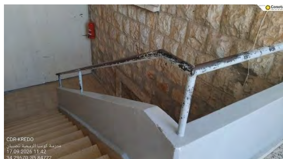
Figure 19 - Damaged Handrail Paint
