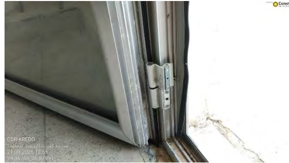
Figure 21 - Damaged Aluminum Door Accessories
