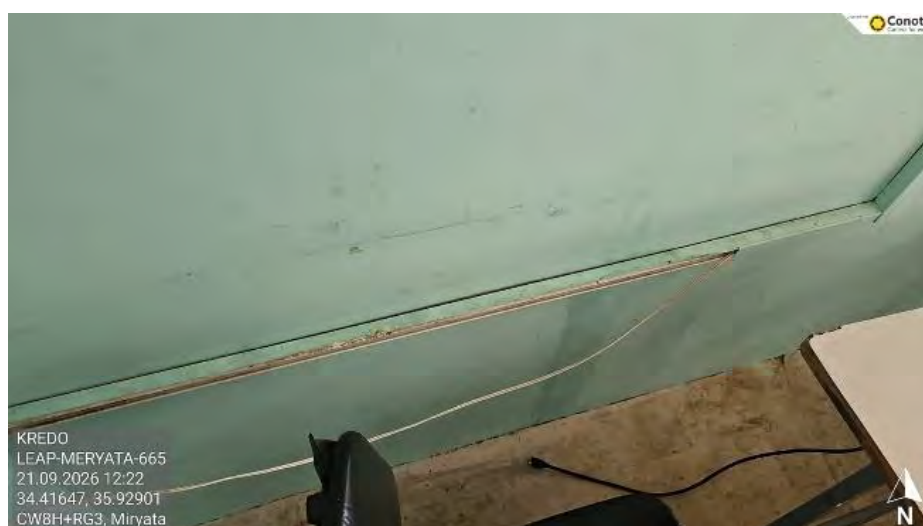
Figure 12 – Damaged Cable Cover
