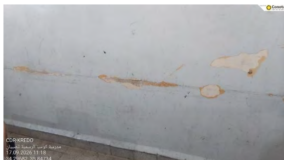
Figure 18 - Damaged Wall Paint
