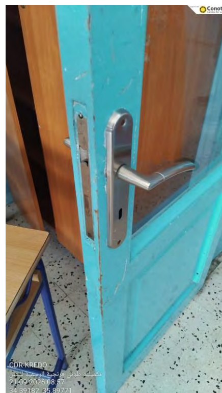
Figure 20 - Door Lock not in good condition
