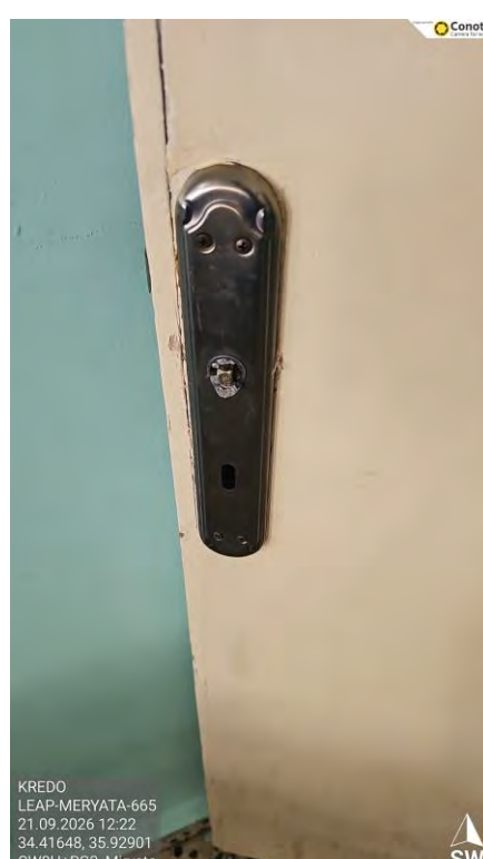
Figure 10 – Damaged Door Handle
