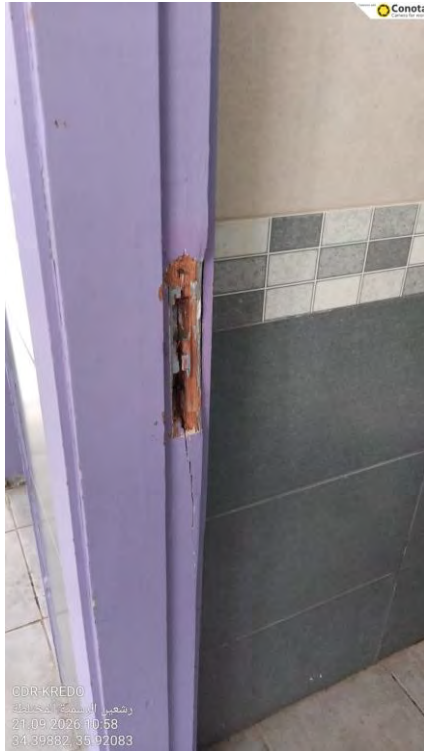
Figure 16 - Damaged Door Accessories
