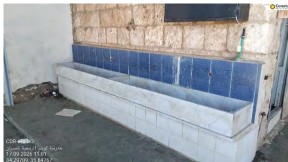
Figure 14 - Missing Drinking Taps
