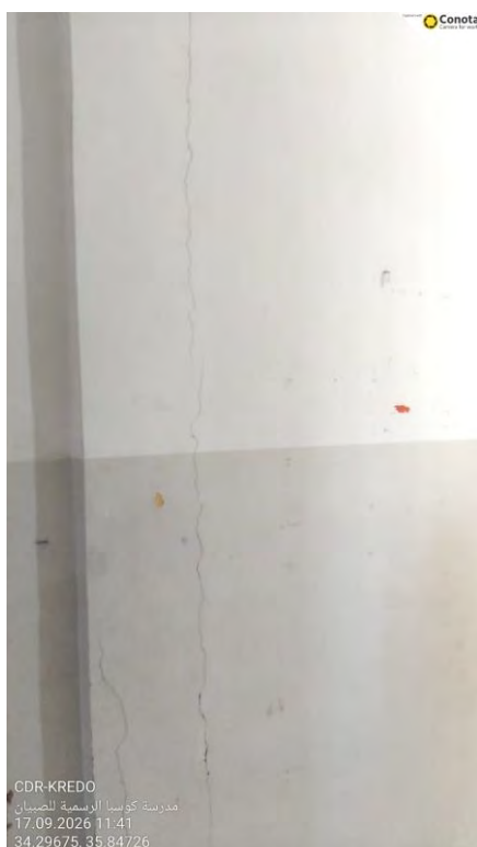
Figure 12 - Crack in Wall
