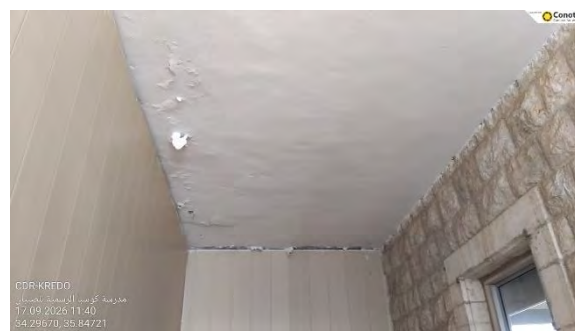
Figure 6 - Humidity in Ceiling
