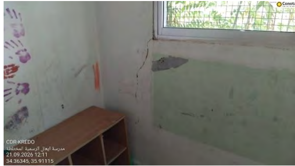
Figure 10 - Crack in wall
