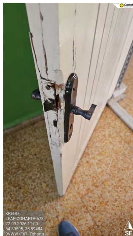
Figure 14 – Damaged Door Handle
