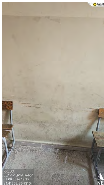
Figure 13 – Damaged Wall Paint
