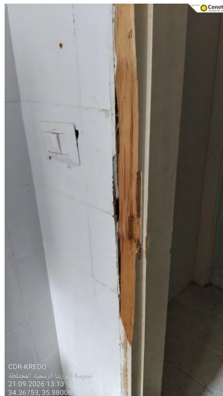
Figure 11 - Broken Door Frame
