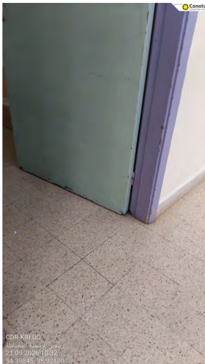
Figure 18 - Damaged Door Paint
