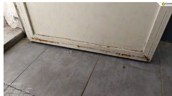
Figure 15 - Rusty Steel Door
