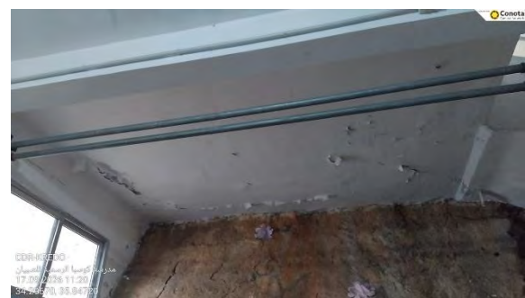
Figure 7 - Humidity in Ceiling
