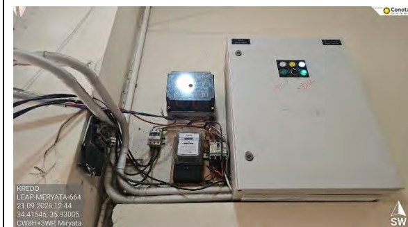
Figure 9 – Unprotected Electrical Installation
