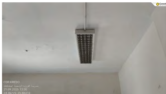
Figure 16 - Damaged Lighting fixture
