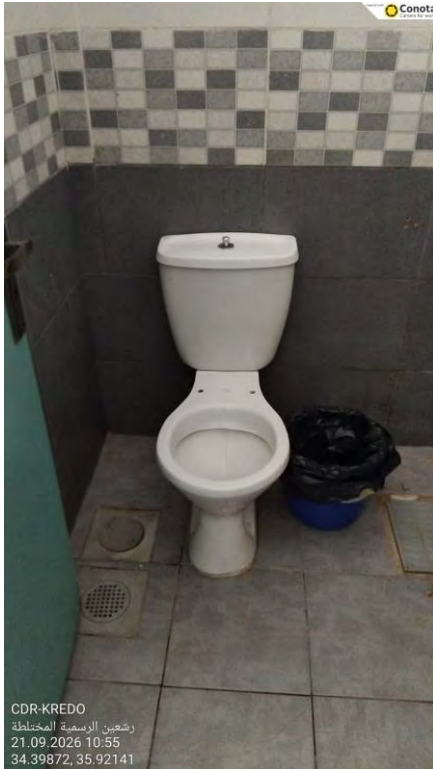
Figure 10 - Missing Toilet Seat Cover
