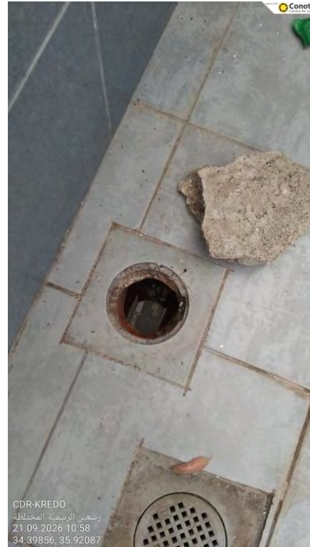
Figure 11 - Missing Manhole Cover
