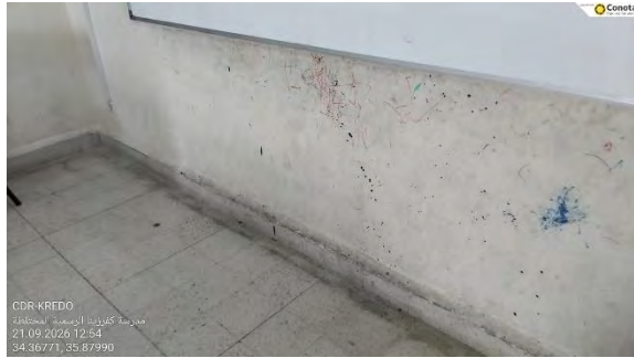
Figure 20 - Damaged Wall Paint
