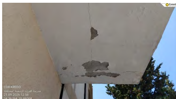
Figure 18 - Damaged Balcony Roof
