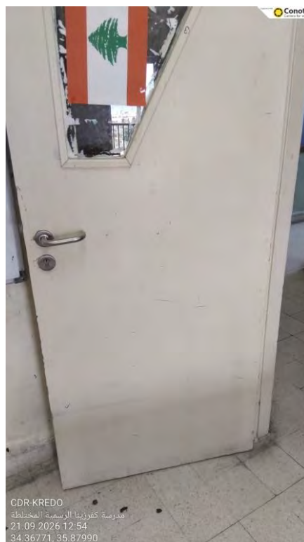
Figure 22 - Damaged Door Paint
