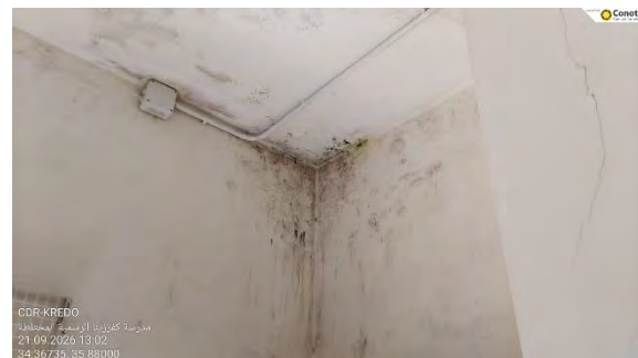
Figure 15 - Humidity in Wall
