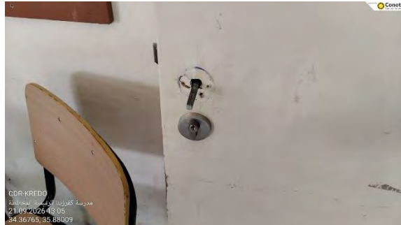
Figure 12 - Missing Door Handle
