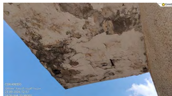
Figure 19 - Spalled Concrete with Exposed Reinforcement
