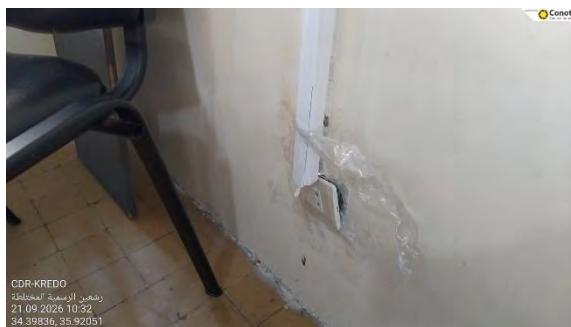
Figure 12 - Damaged Electrical Socket
