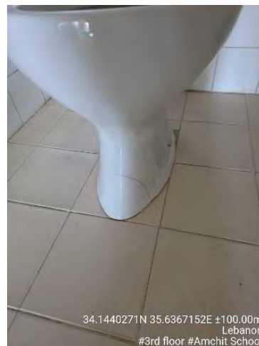
Figure 8- Broken Toilet Seat
