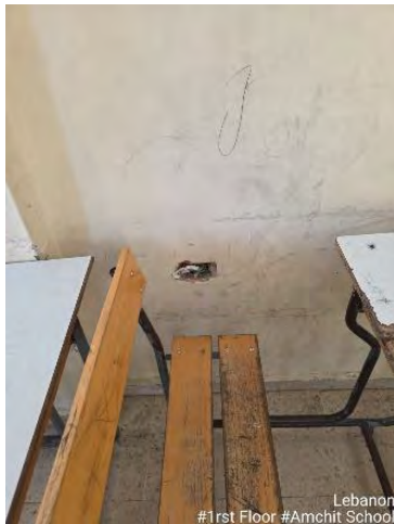
Figure 11- Damaged Electricity Socket
