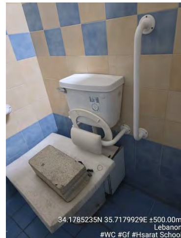
Figure 8- Broken Toilet Seat
