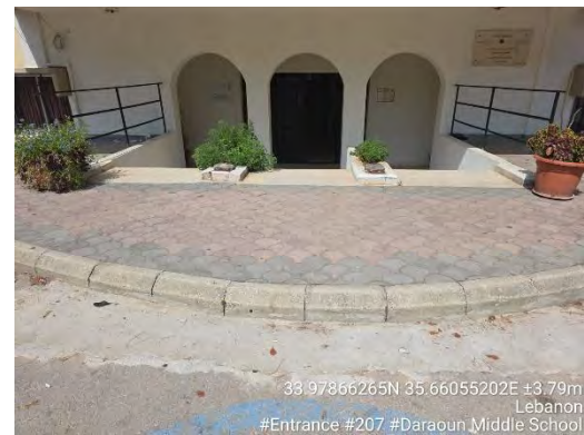
Figure 10- Handrail need painting
