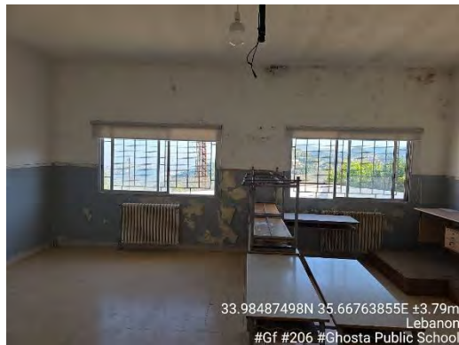
Figure 5- Ceiling & Walls in bad condition
