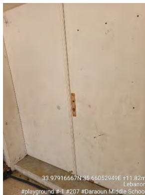
Figure 9- Missing door accessories
