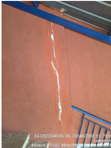
Figure 10- Crack in Columns
