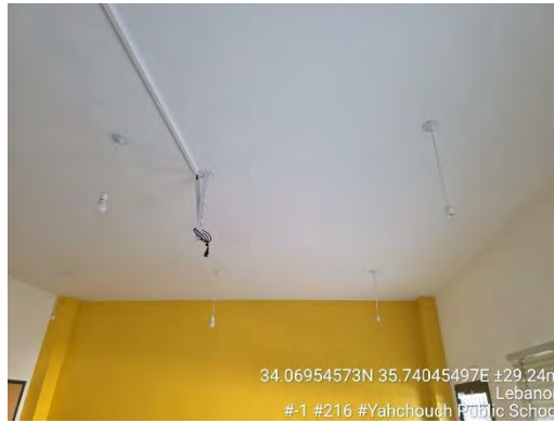
Figure 13- Missing light bulbs
