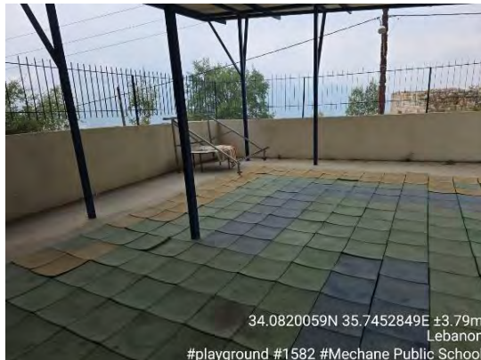
Figure 6- Playground in bad conditions
