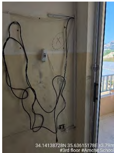
Figure 5- Electrical wires to be properly installed
