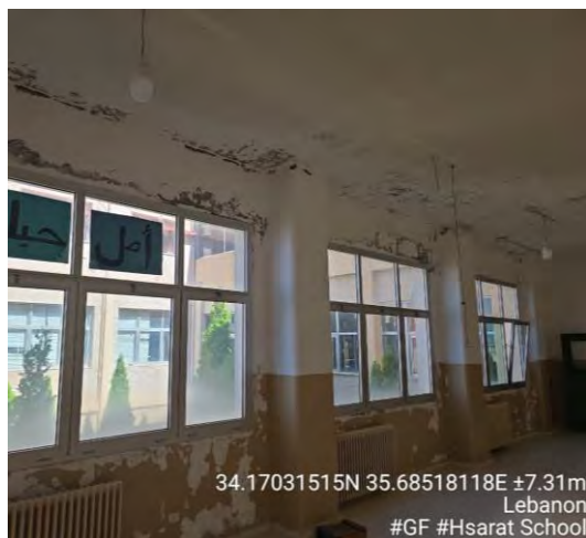
Figure 9- Damaged Walls Due to Water Leakage
