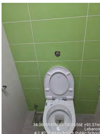
Figure 9- Damaged Sanitary Accessories
