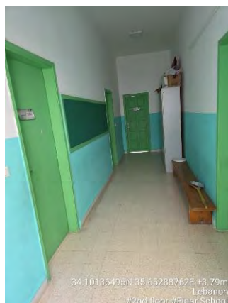
Figure 6- Walls, Ceiling and Doors in bad condition
