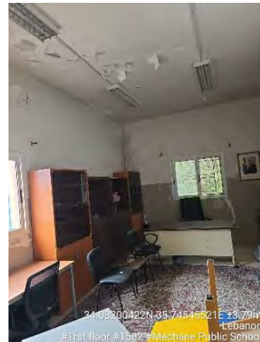
Figure 5- Walls, Ceiling and doors in bad condition
