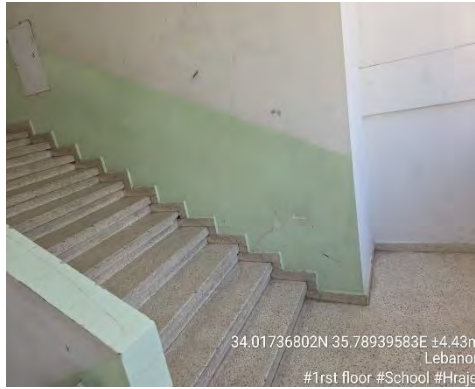
Figure 12- Cracks in staircase
