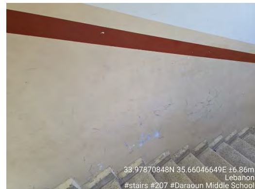
Figure 12- Cracks in staircase
