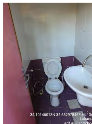
Figure 7- Toilet door with deteriorated paint finish and damaged accessories
