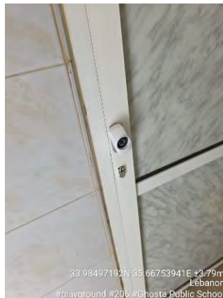
Figure 7- Damaged Door accessories
