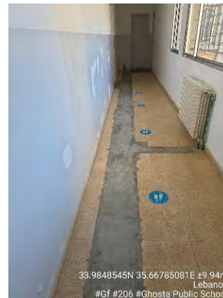
Figure 8- Damaged Tiles due to pipe replacing for shelter use
