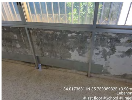
Figure 10- Wall paint in bad condition
