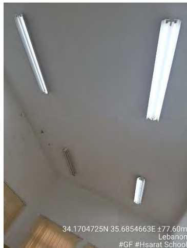
Figure 7- Damaged Lighting Fixtures
