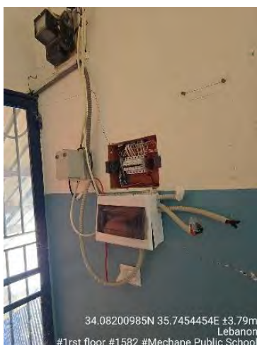
Figure 8- Electrical panel in bad condition along with visible shear crack
