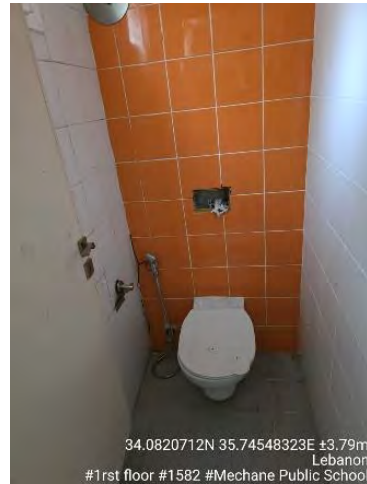
Figure 11- Damaged Toilet Seat
