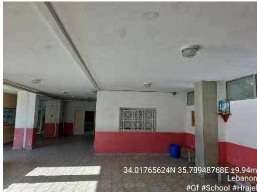
Figure 6- Damaged Wall Paint
