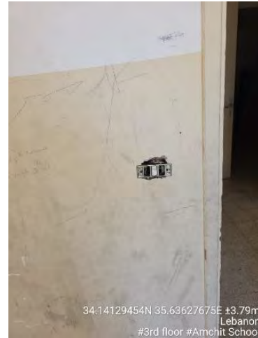
Figure 10- Damaged Electricity Switch
