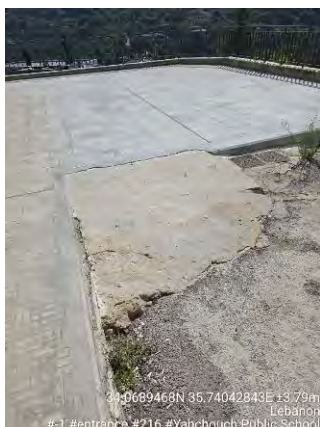
Figure 7- Ramp in bad condition
