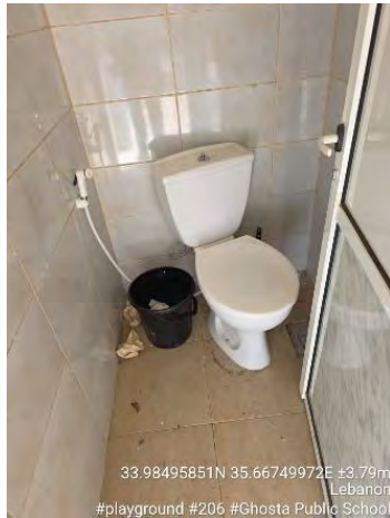
Figure 11- Damaged Toilet Seat
