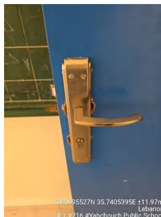
Figure 8- Damaged door's handle
