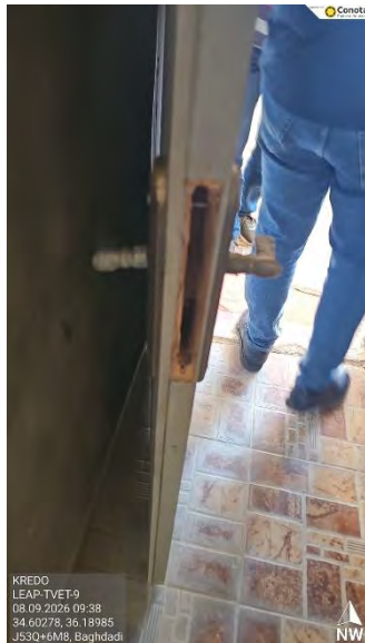
Figure 15- Door Handles in bad condition
