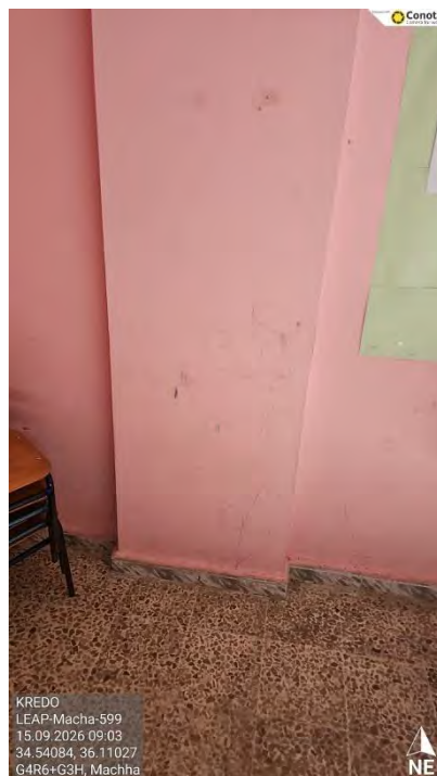
Figure 8 - Paint in Bad condition
