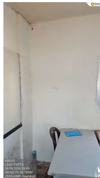
Figure 10- Paint in bad condition
