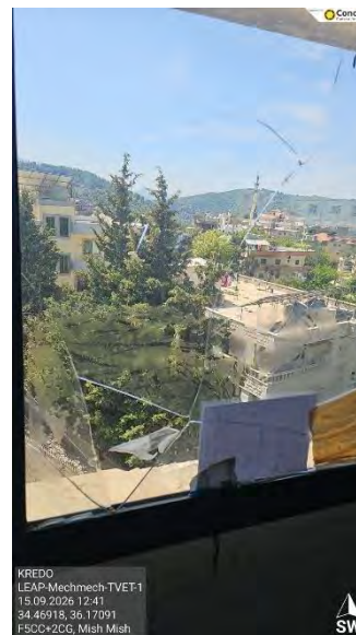
Figure 12 - Cracked Window Glazing
