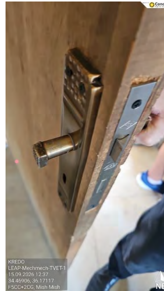
Figure 10 - Damaged Door Handle
