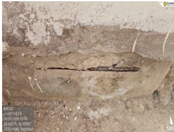
Figure 7- Spalled concrete with exposed reinforcement.
