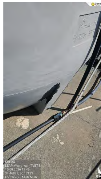
Figure 16 - water Tank Leakage
