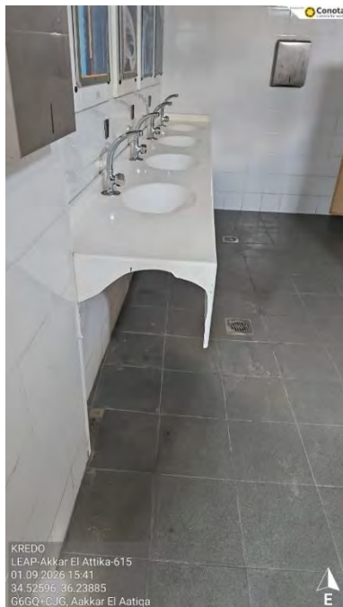
Figure 6 – Damaged Wash Basin
