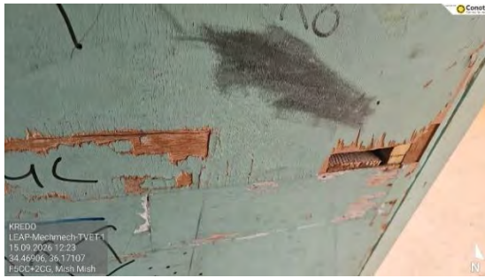
Figure 7 - Doors in Bad Condition
