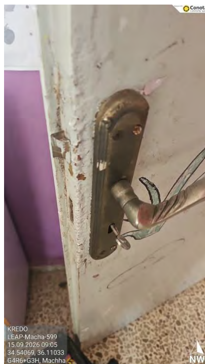
Figure 14 - Door Handles in bad condition
