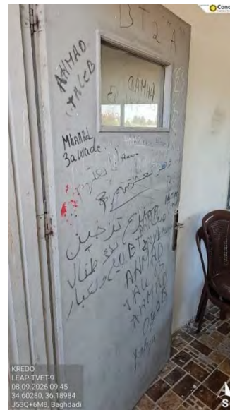
Figure 8- Doors in bad condition
