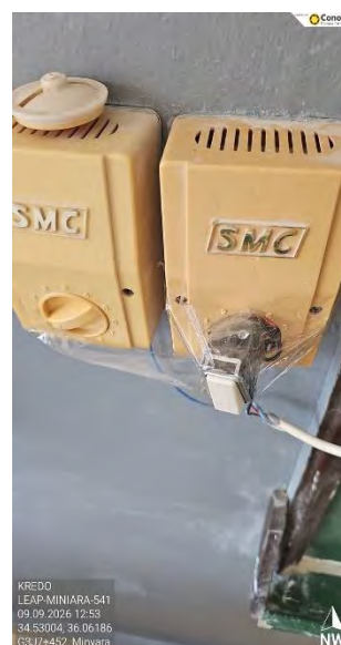
Figure 9 – Damaged Fan Switches
