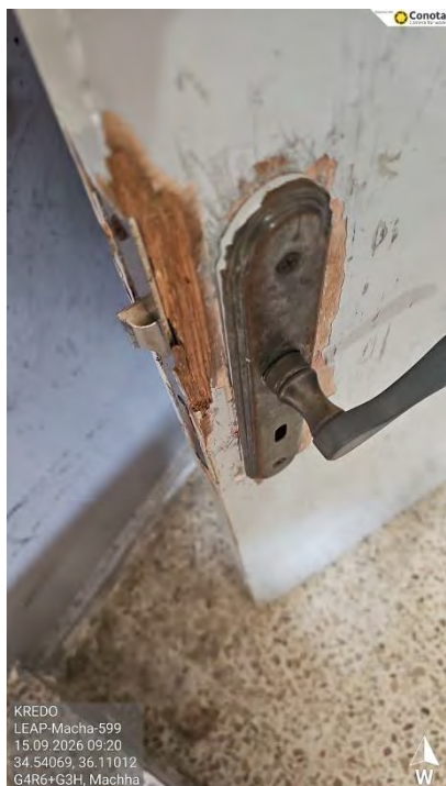
Figure 7 - Doors in bad condition
