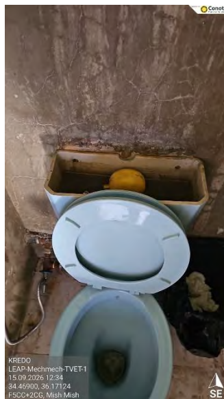
Figure 11 - Damaged Toilet seat
