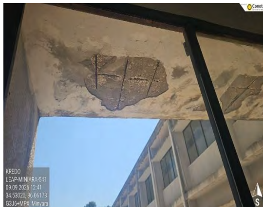
Figure 4 – Spalled concrete with exposed reinforcement
