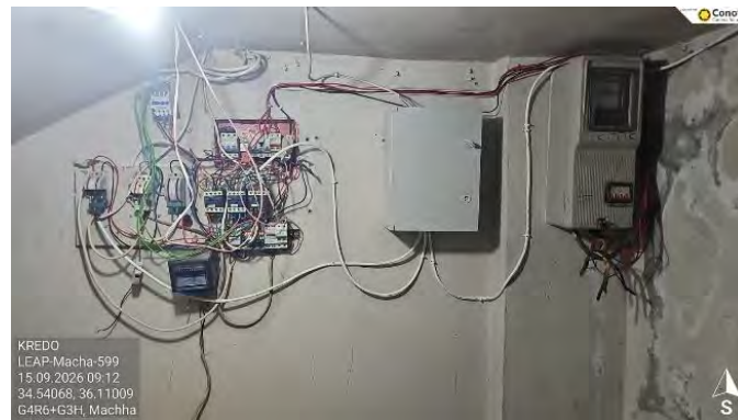
Figure 15 – Unprotected electrical installation
