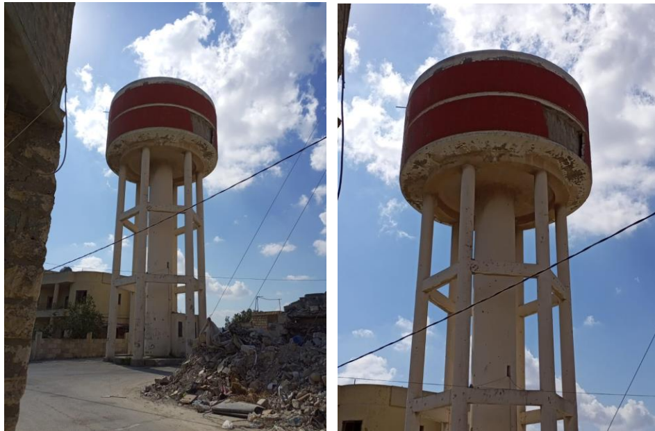
S2-2 — Elevated water tank (33.26082, 35.41960)
