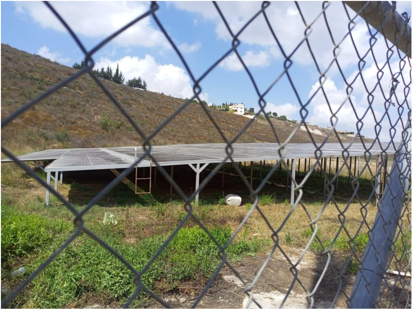
S2-1 — Solar pumping system (33.25854, 35.41270)
