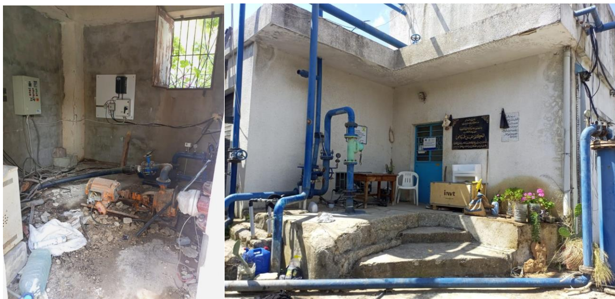
S2-5 — Water pumping station (33.24793, 35.41974)
