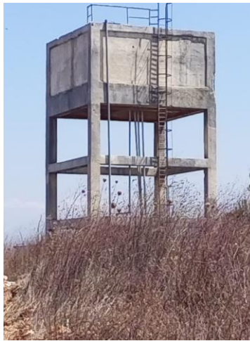
S2-3 — elevated reservoir standing but showing cracks
