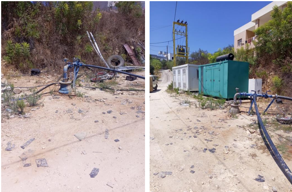
S2-3 — Village water well and pumping station (33.27639, 35.39294)
