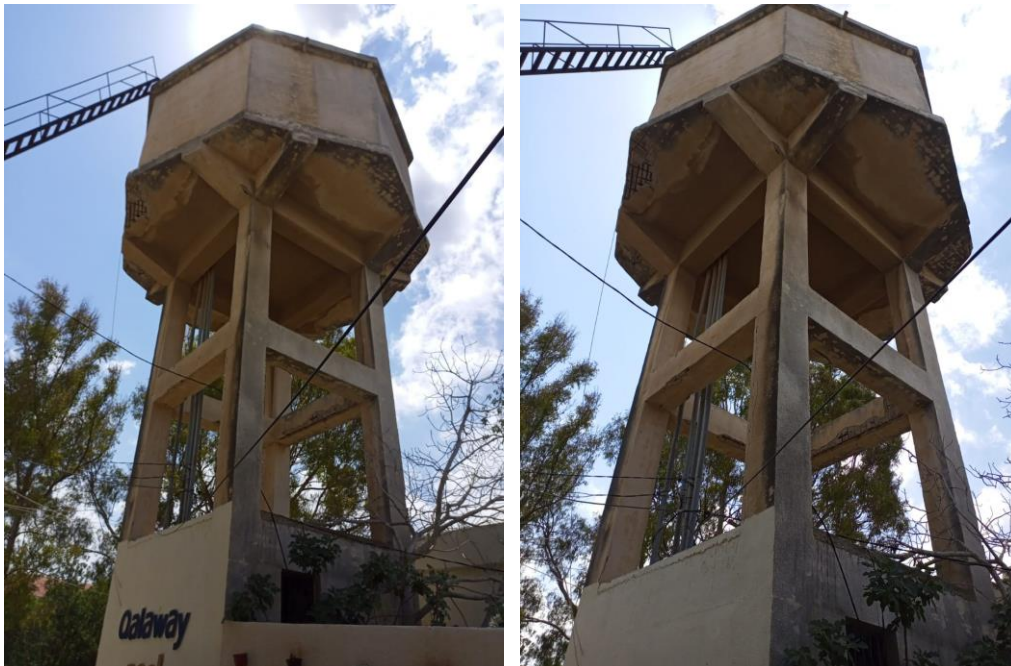
S2-4 — Elevated water tank (33.24793, 35.41974)
