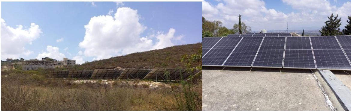
S2-3 — Solar array for the sub-network pump (33.24793, 35.41974)
