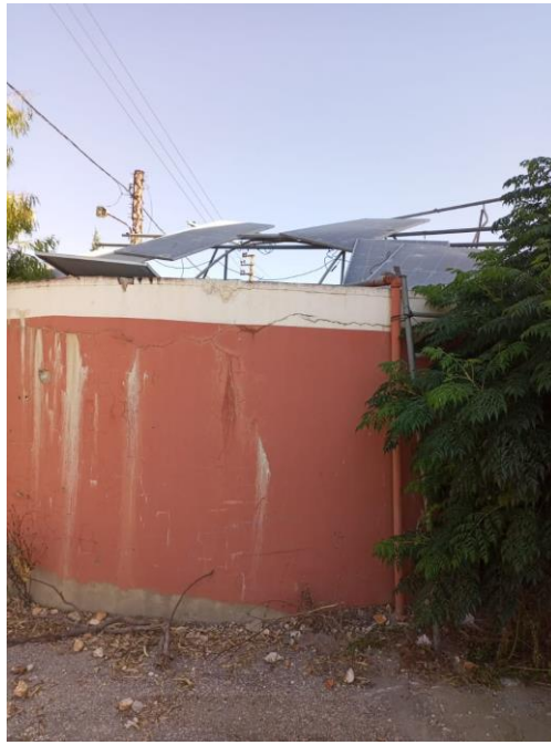
S2-5 — Solar array — booster/treatment station (33.29144, 35.42947)
