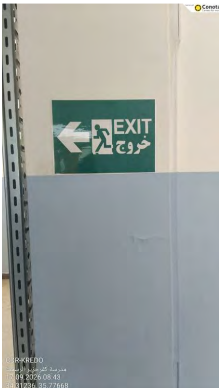
Figure 11 - Damaged Wall Paint
