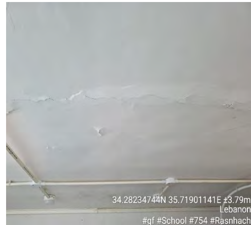
Figure 6- Damaged plaster due to water leakage
