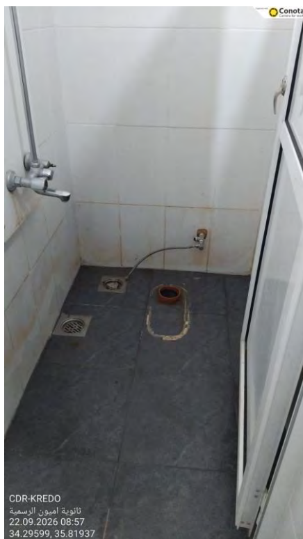
Figure 13 - Missing Toilet Seat
