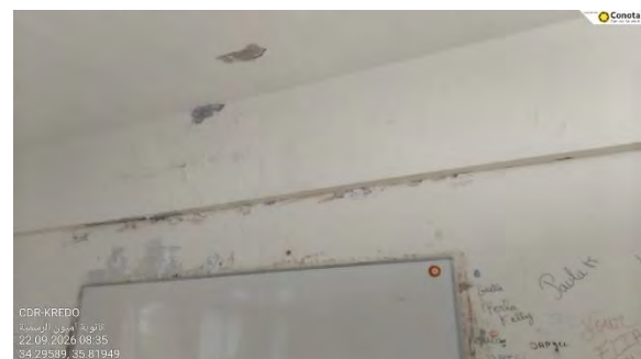
Figure 8 - Humidity in Wall
