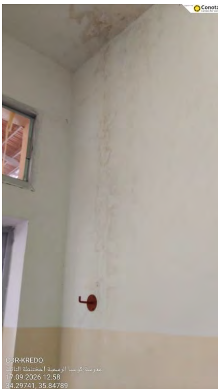
Figure 12 - Humidity in Wall & Ceiling
