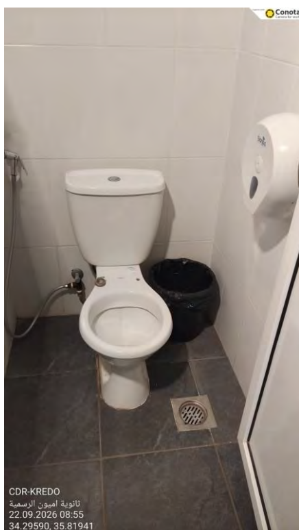
Figure 15 - Missing Toilet Seat Cover
