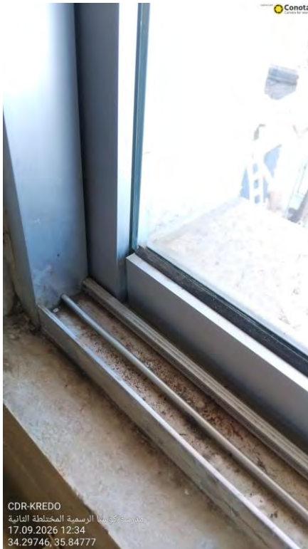
Figure 10 - Broken Aluminum Window
