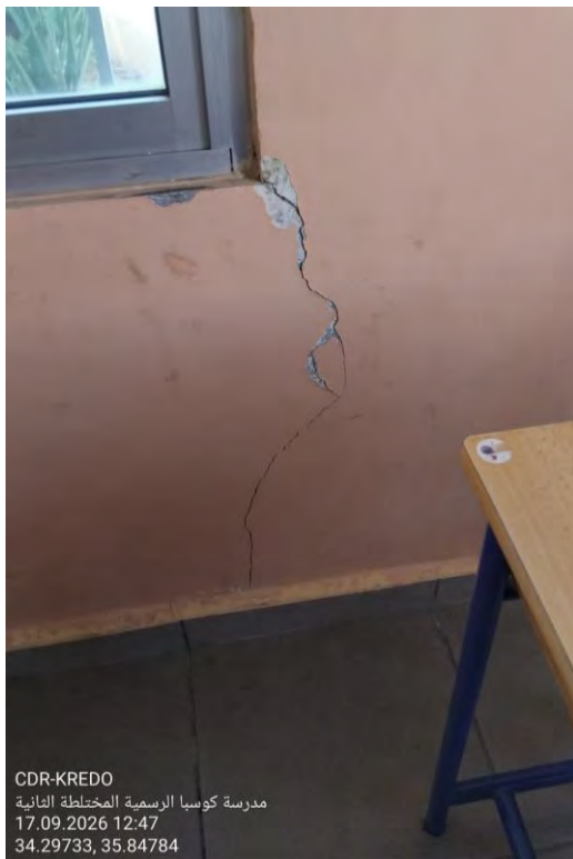
Figure 16 - Crack in Wall
