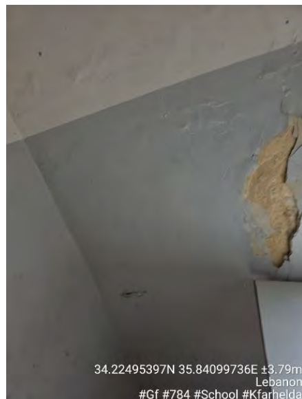
Figure 8- Damaged plaster due to water leakage
