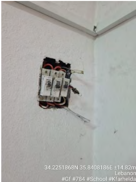
Figure 9- Electrical panel damaged
