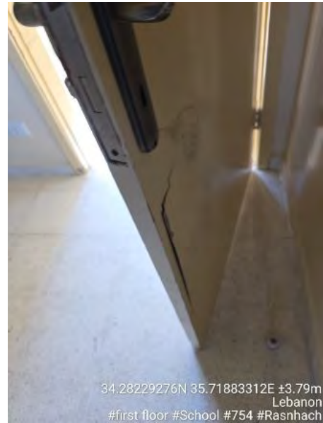
Figure 10- Damaged Wooden Door
