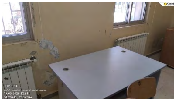
Figure 6 - Damaged Wall Paint
