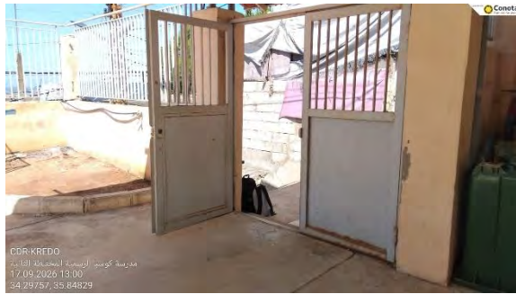
Figure 14 - Rusty Main Gate
