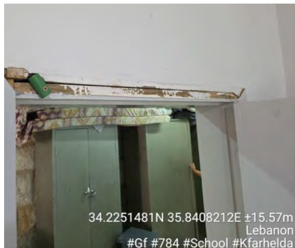
Figure 13- Damaged wooden door
