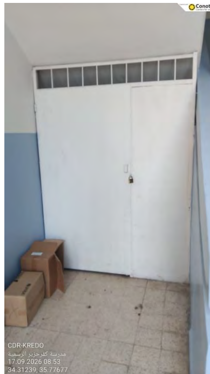
Figure 10 - Damaged Steel Door Paint
