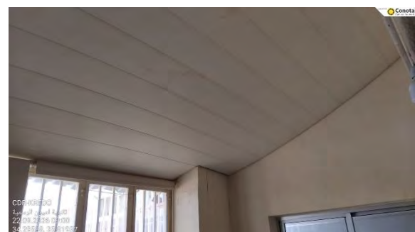
Figure 12 – Damaged False Ceiling Leveling
