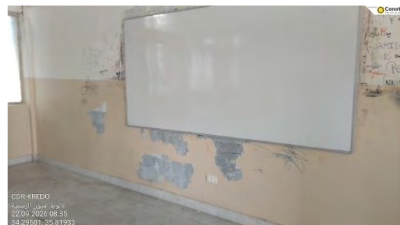
Figure 9 - Damaged Wall Paint
