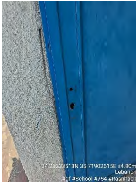
Figure 9- Steel door accessories damaged
