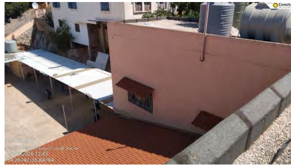
Figure 15 - Crack in Elevation
