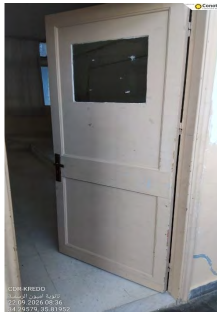
Figure 20 - Damaged Door Paint
