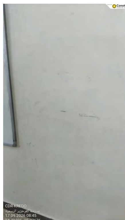
Figure 8 - Damaged Wall Paint
