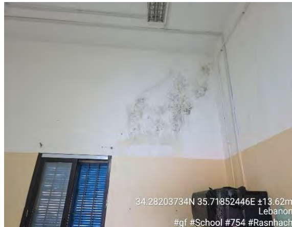
Figure 5- Ceiling & walls in bad condition
