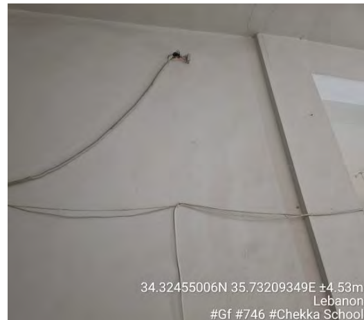
Figure 6- Electrical wires to be properly installed
