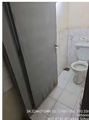
Figure 10- Damaged Wooden Door
