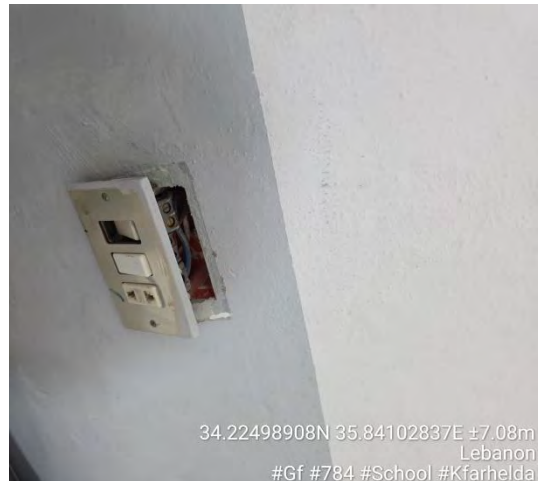
Figure 6- Electrical switch damaged
