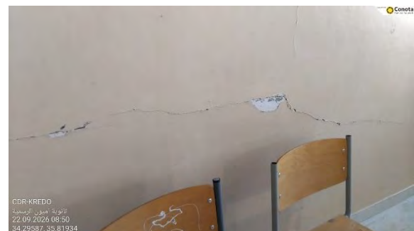
Figure 10 - Crack in Wall
