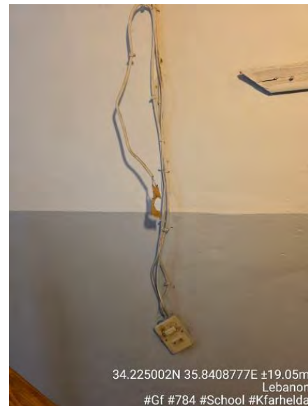
Figure 12 - Electrical wires to be properly installed
