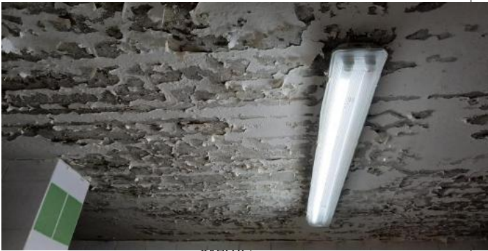
Humidity and water leak from the roof and elevations shown inside the building
