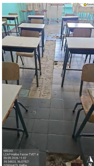
Figure 9 – Damaged Floor Tiles
