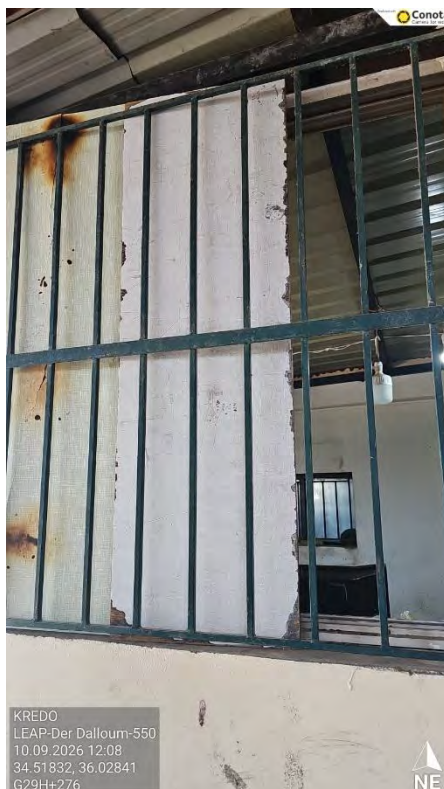
Figure 12 -Window glazing in bad condition
