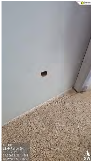
Figure 7 - Doors in bad condition
