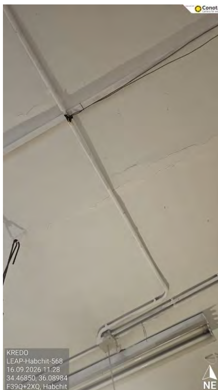
Figure 9 - Roof Slab Cracks (1)
