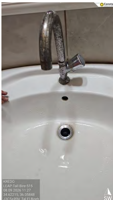
Figure 4 – Mixers in bad condition
