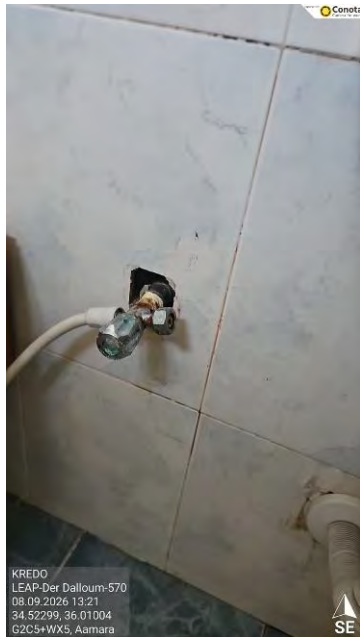
Figure 4 – Damaged Angle Valve
