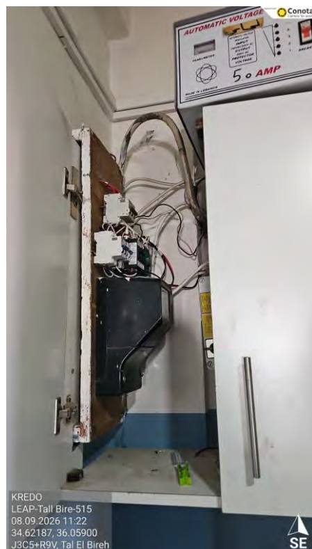
Figure 13 - Unprotected electrical installation
