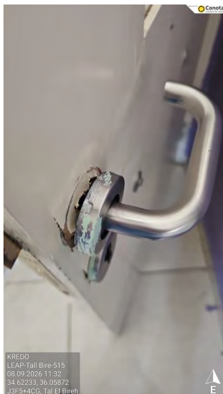
Figure 12 - Damaged door handle
