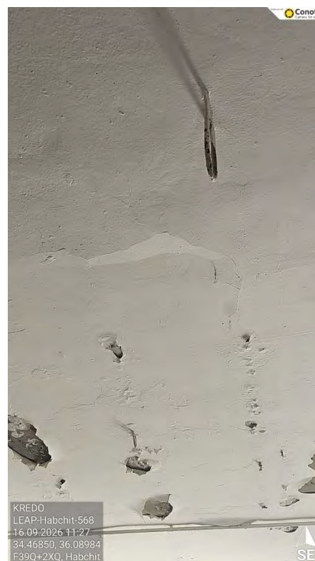
Figure 10 - Roof Slab Cracks (2)
