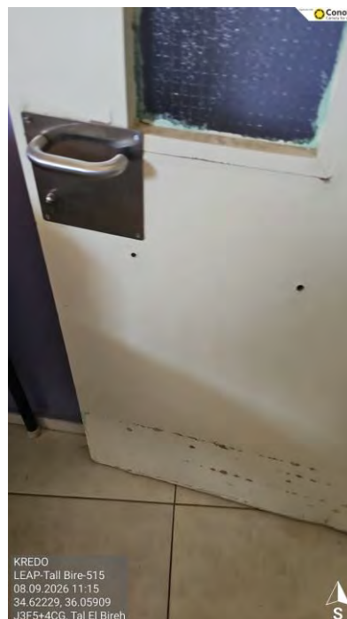
Figure 5 - Damaged door paint
