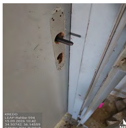
Figure 14 - Door Handles in bad condition
