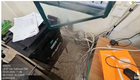
Figure 8 – Unprotected electrical installation
