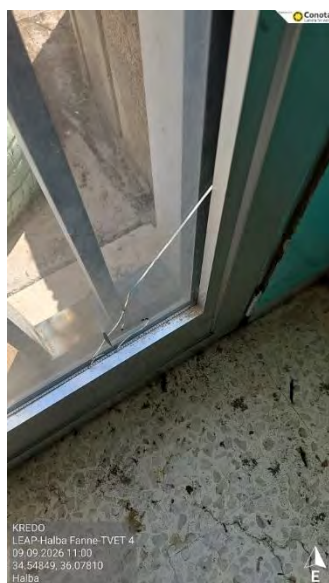
Figure 13 – Damaged Door Glazing
