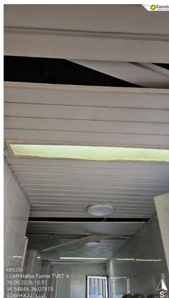
Figure 7 – Damaged False Ceiling
