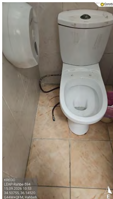
Figure 11 - Damaged toilet seat
