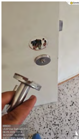
Figure 12 - Broken Door Handle
