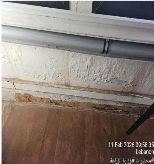
Water leakage from aluminum opening
