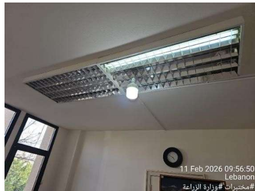
Lighting to be rehabilitated
