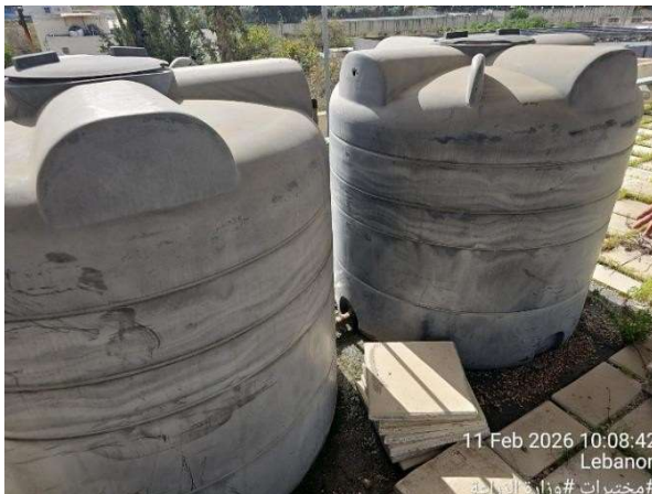
Water tanks to be replaced
