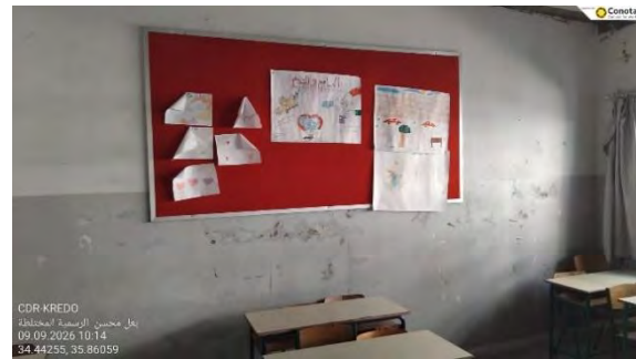
Figure 15 – Damaged Wall Paint
