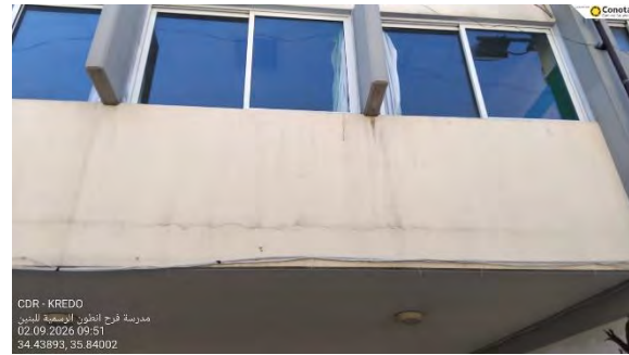
Figure 21 - Humidity in External Wall
