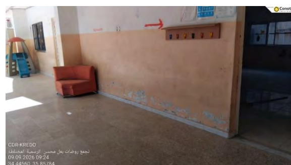
Figure 11 – Damaged Wall Paint
