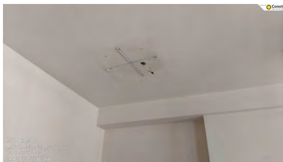
Figure 8 – Missing Light Fixture
