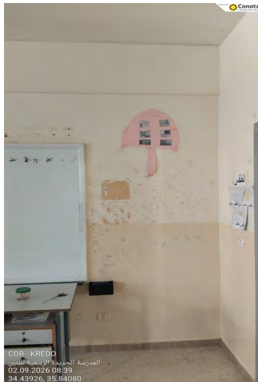
Figure 8 – Damaged Wall Paint
