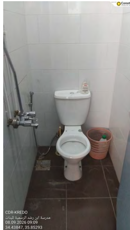
Figure 9 – Missing Toilet Seat Cover
