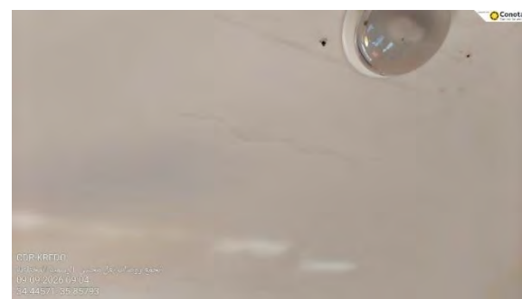
Figure 7 – Cracks in Ceiling
