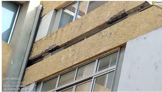
Figure 16 – Exposed Rebars at Elevation
