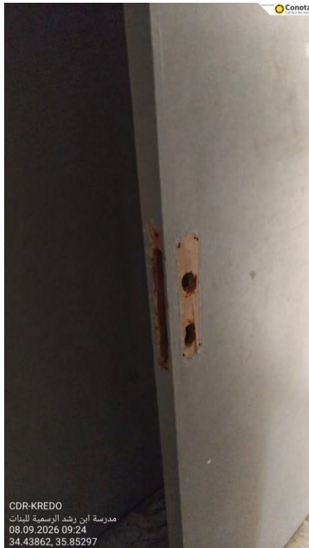
Figure 8 – Missing Door Handle & Lock
