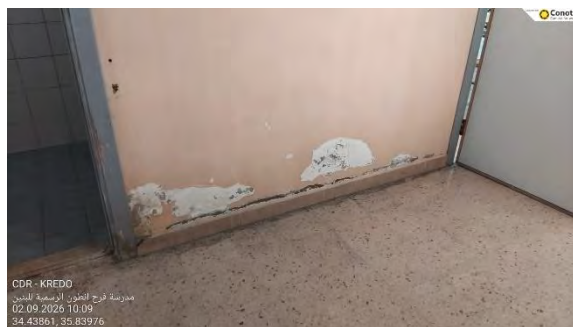
Figure 16 - Humidity in Wall
