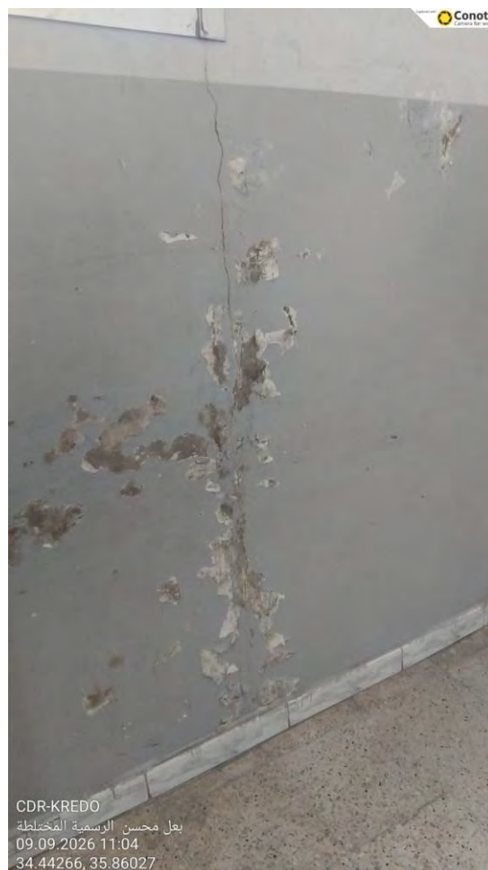
Figure 11 – Cracks in Wall
