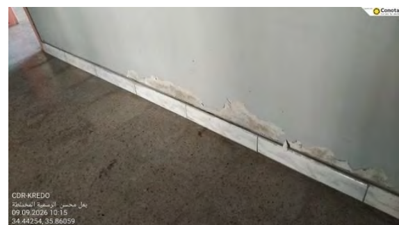
Figure 19 - Humidity in Wall
