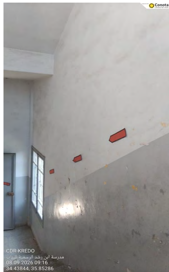
Figure 15 – Damaged Wall Paint
