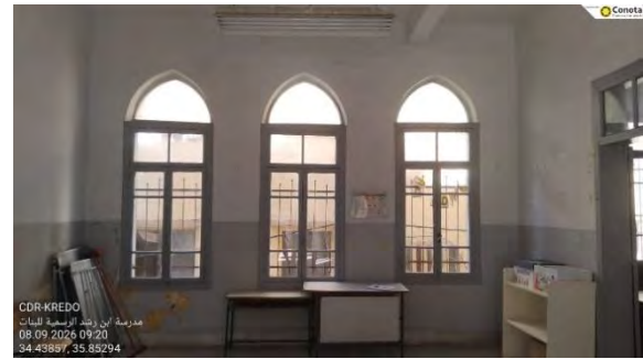
Figure 13 – Damaged Wall Paint
