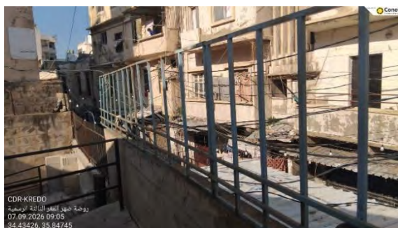
Figure 10 – Rusty Steel Fence
