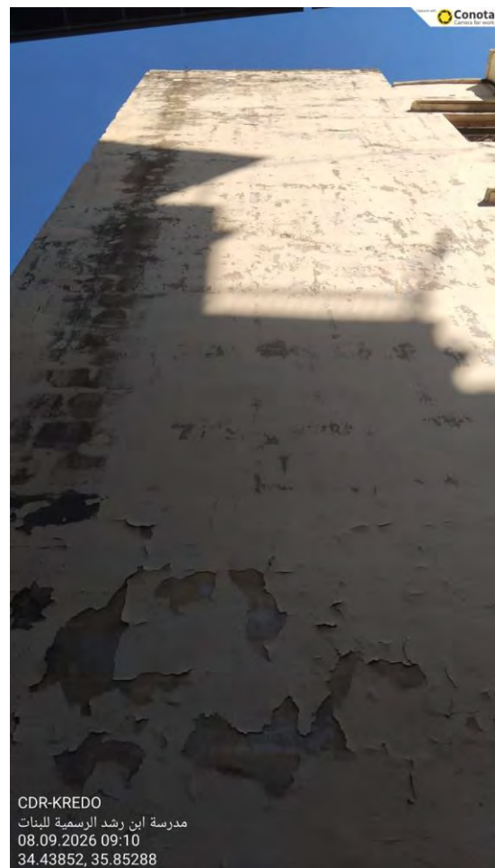
Figure 7 – Damaged Exterior Wall
