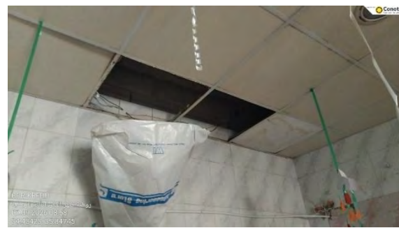
Figure 5 – Missing False Ceiling Boards
