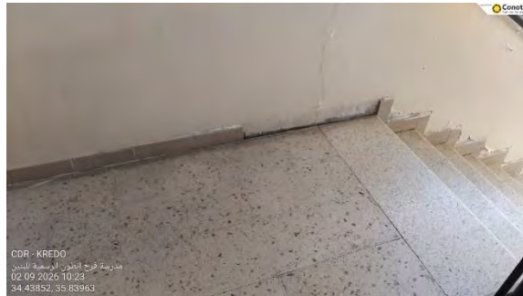
Figure 14 – Crack in Wall
