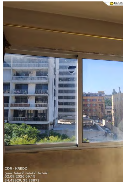
Figure 9 – Broken Window Glass
