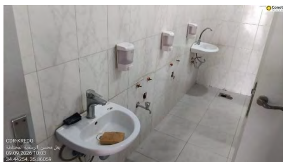
Figure 12 – Missing Wash Basins
