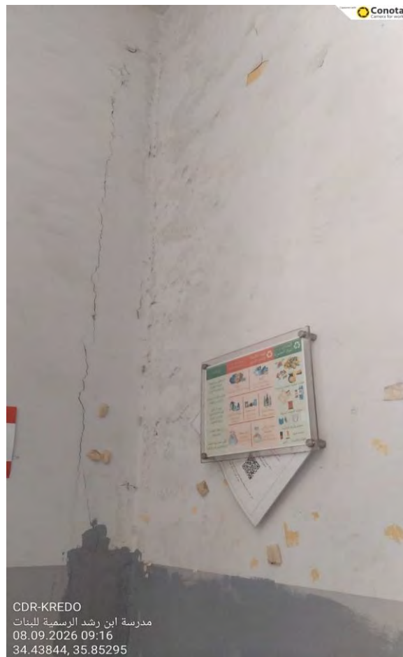
Figure 14 – Crack in Wall
