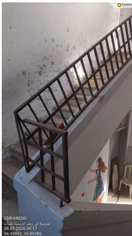
Figure 10 – Rusted Stair Handrail
