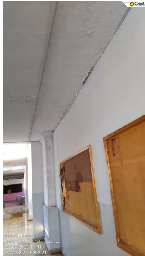
Figure 17 - Humidity in Wall
