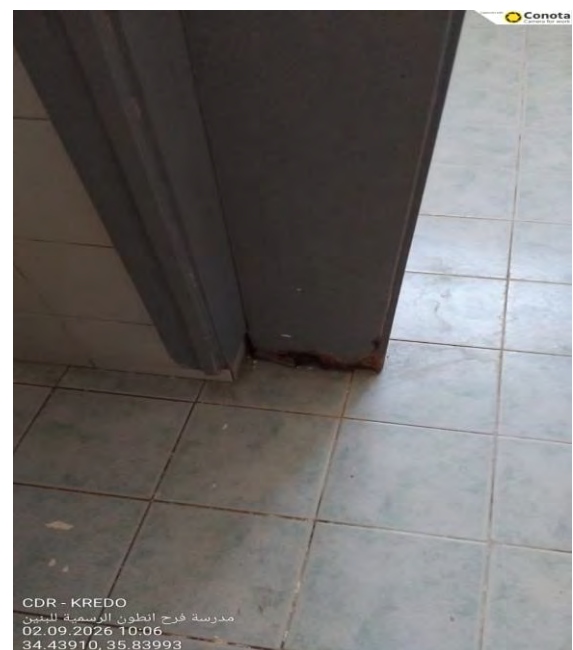
Figure 18 - Damaged Door Frame
