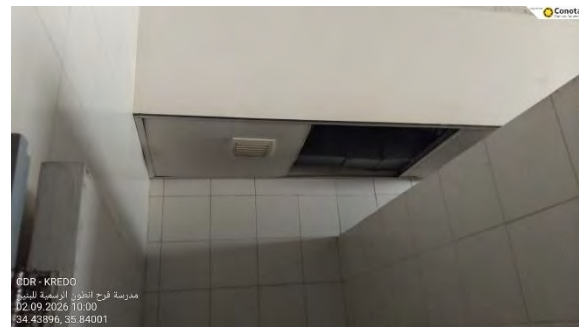
Figure 23 - Damaged False Ceiling
