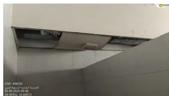
Figure 11- Damaged False Ceiling
