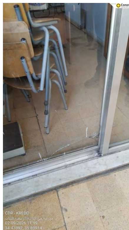
Figure 11 – Broken Door Glazing
