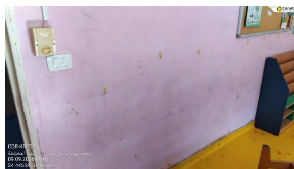
Figure 6 -Damaged Wall Paint
