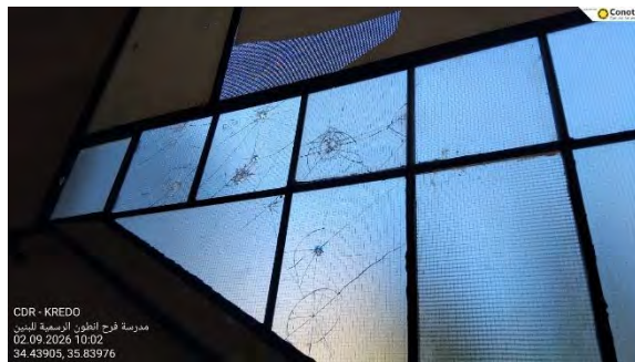
Figure 22 - Broken Window Glazing
