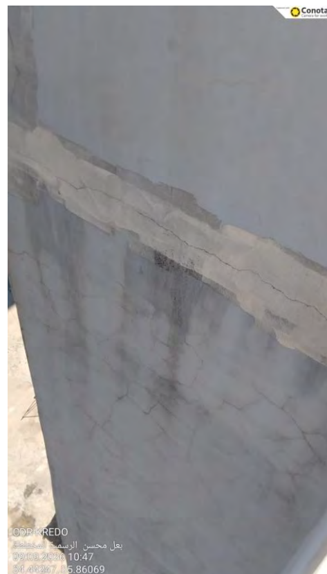
Figure 9 – Cracks in Elevation
