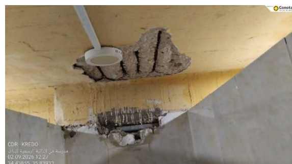
Figure 14 – Exposed and Rusted Rebars
