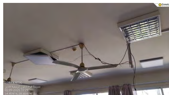
Figure 9 – Damaged Electrical Wiring
