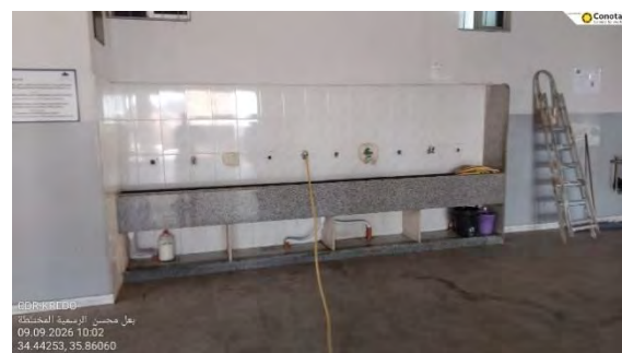
Figure 7 – Missing Drinking Taps
