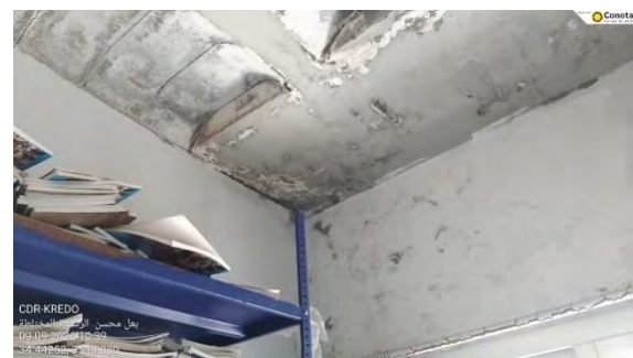
Figure 17 - Humidity in Roof
