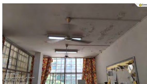
Figure 7 – Humidity in Roof
