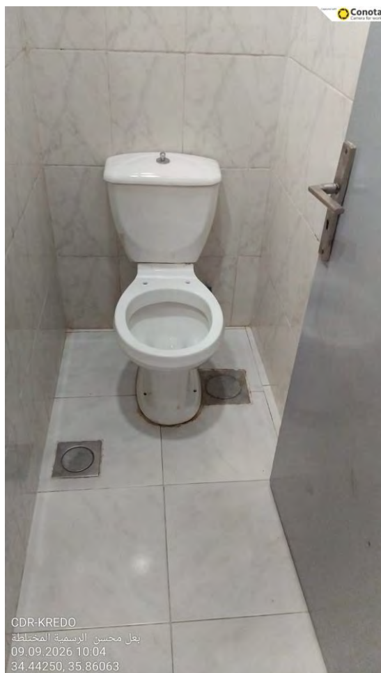
Figure 10 – Missing Toilet Seat Cover
