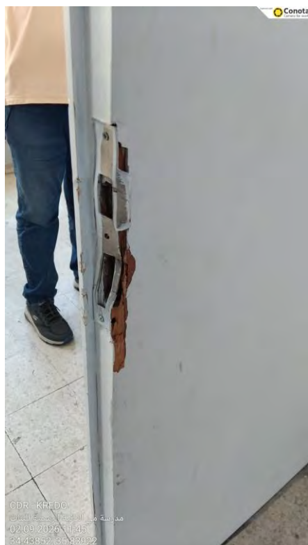
Figure 10 – Damaged Door Accessories
