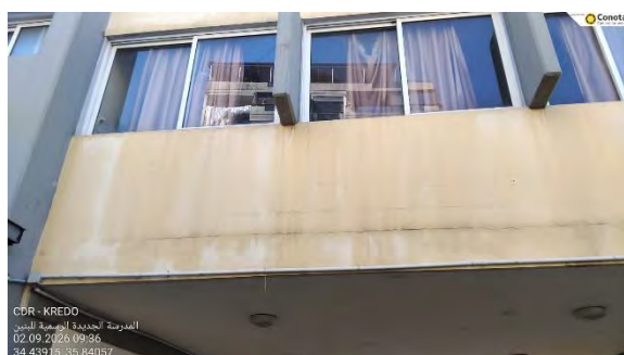
Figure 14 – Humidity in External Wall
