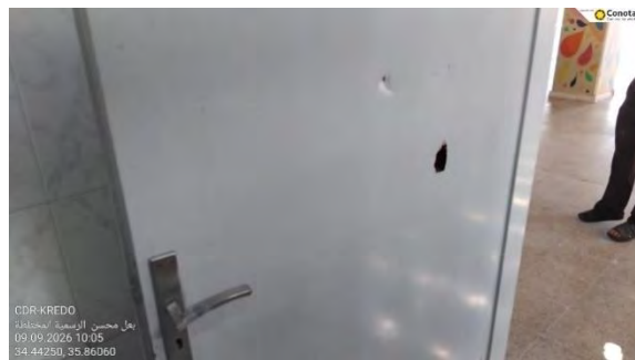
Figure 16 – Damaged Timber Door
