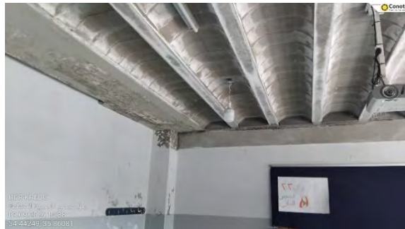
Figure 14 – Humidity in Roof
