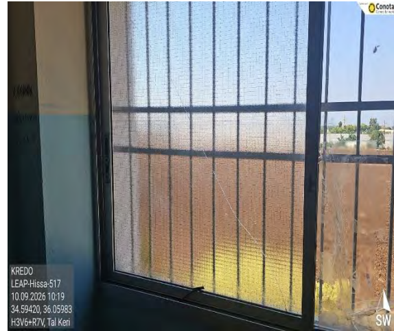
Figure 13 - Unprotected Electrical Installation
