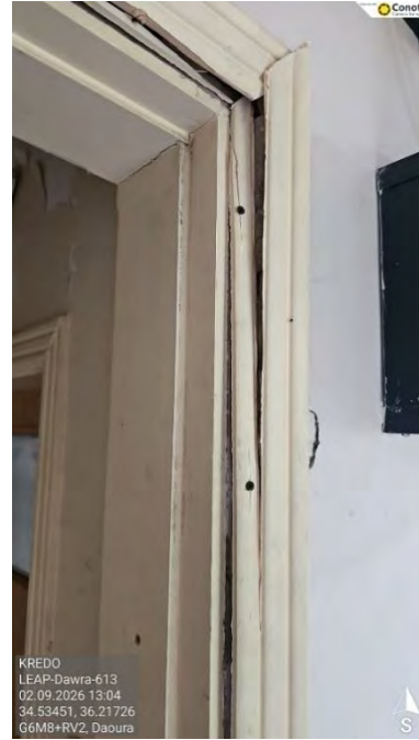
Figure 7 – Damaged Door Frames
