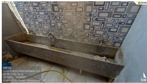
Figure 10 – Damaged Water Taps
