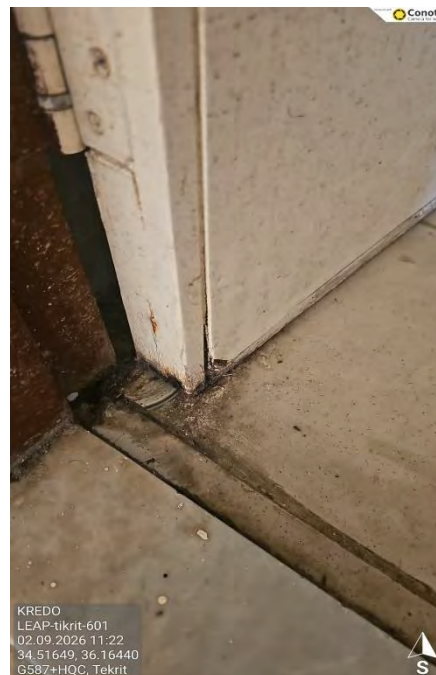
Figure 7 – Damaged Wooden Doors
