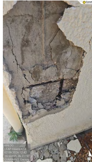
Figure 9 – Spalled Concrete with Exposed Reinforcement
