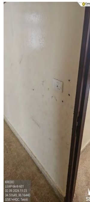
Figure 5 – Damaged Door Frames
