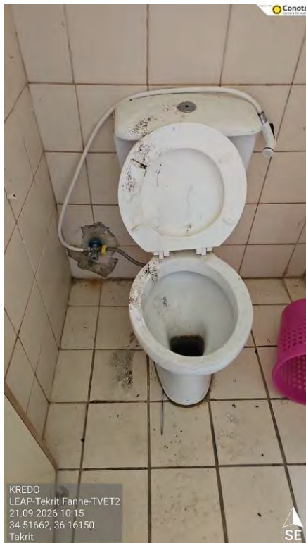
Figure 11 - Damaged Toilet Seat
