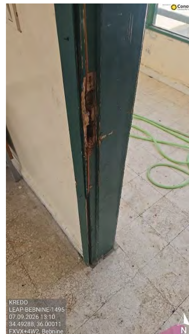
Figure 11 – Damaged door frame
