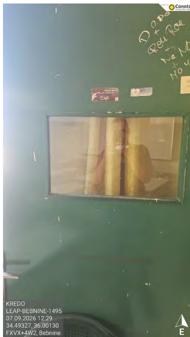
Figure 6 – Damaged door paint
