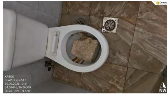
Figure 5 - Damaged Toilet Seat
