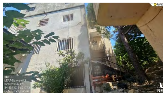
Figure 11 – Spalled Concrete with Exposed Reinforcement
