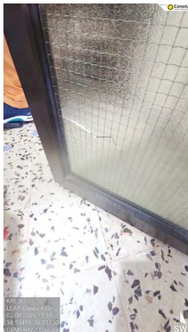
Figure 6 – Damaged Glazed Panel
