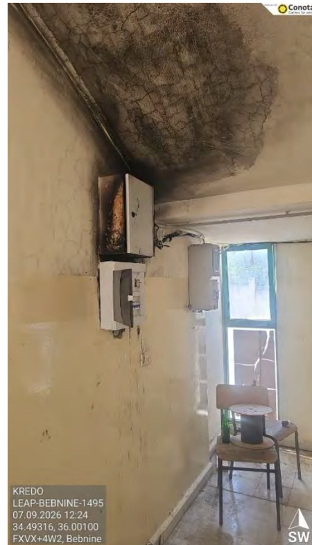
Figure 13 - Unprotected electrical installations and ceiling in poor condition
