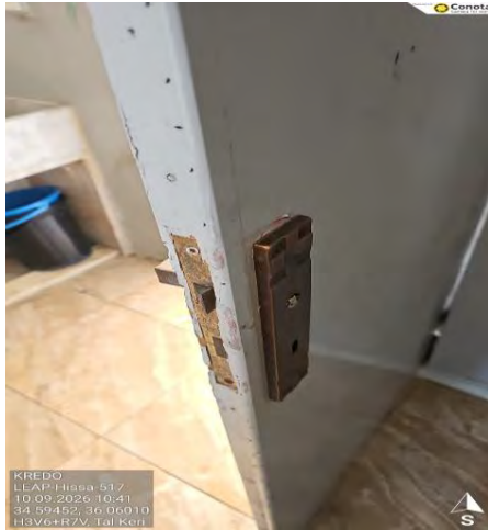
Figure 12 - Damaged Door Handle
