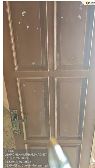
Figure 5 - Damaged Door Paint
