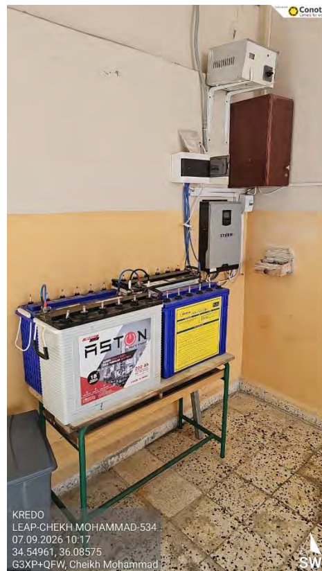
Figure 13 - Unprotected Electrical Installation
