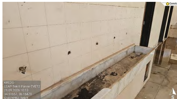
Figure 21 – Damaged Basins and Taps
