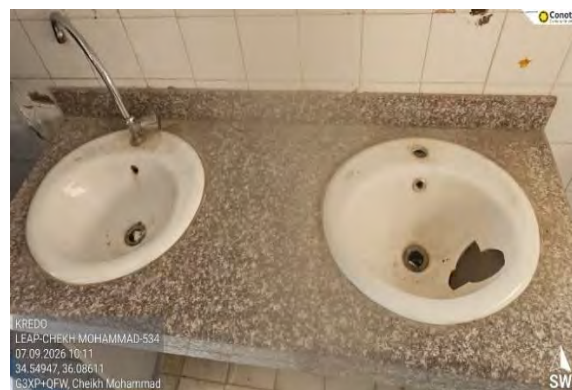
Figure 9 - Damaged Wash Basin
