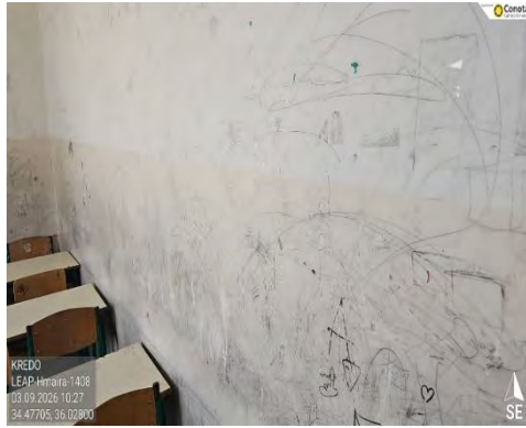
Figure 8 – Damaged wall paint
