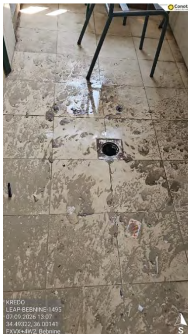
Figure 10 – Damaged floor drain
