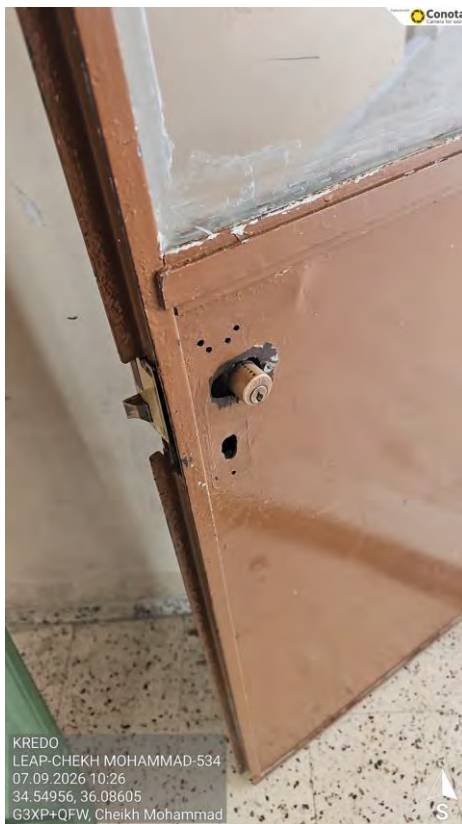
Figure 12 - Missing Door Handle
