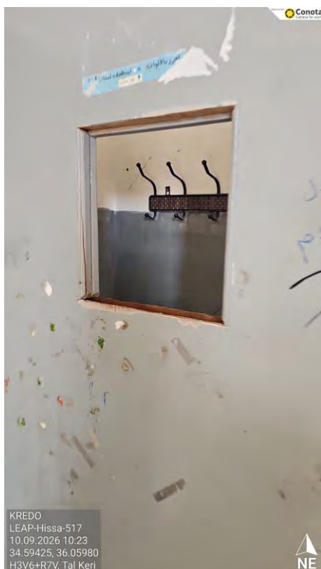
Figure 10 – Damaged Door Glazing
