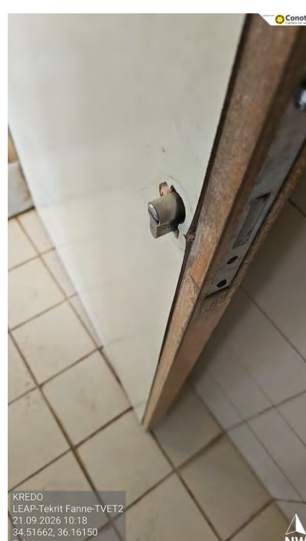
Figure 10 – Damaged Door Handle
