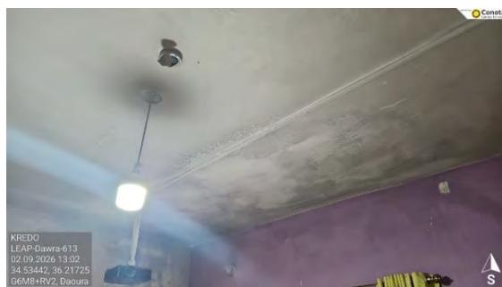
Figure 10 – Damaged Roof Paint
