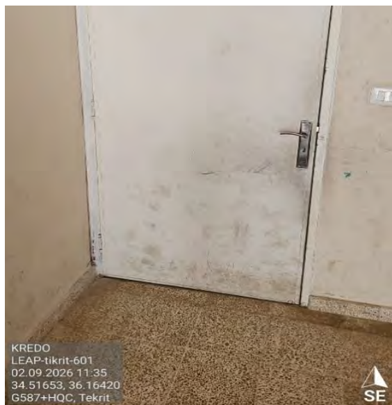
Figure 10 – Damaged Door Paint
