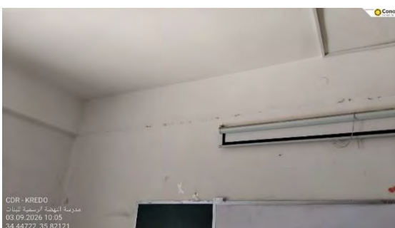
Figure 16 - Crack Between Beam & Wall
