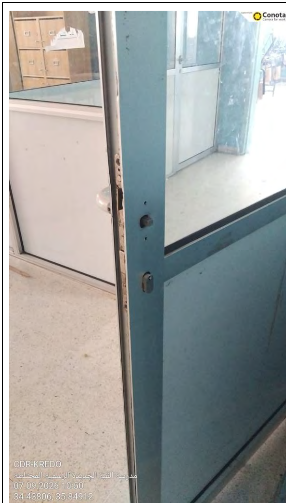
Figure 15 – Missing Door Handle
