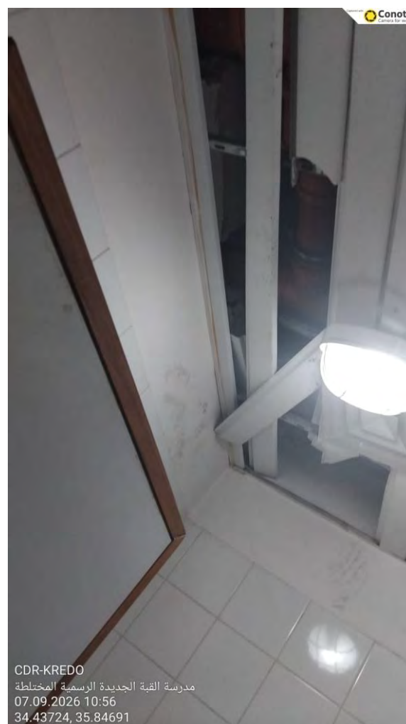
Figure 18 - Damaged False Ceiling
