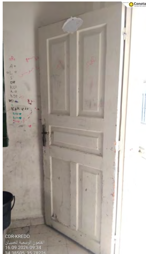
Figure 16 – Damaged Door Paint
