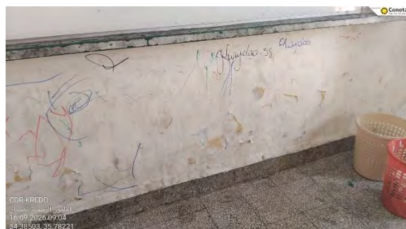
Figure 14 – Damaged Wall Paint
