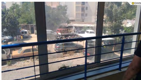
Figure 19 - Broken Window Glazing
