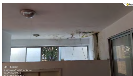
Figure 11 – Humidity in Ceiling
