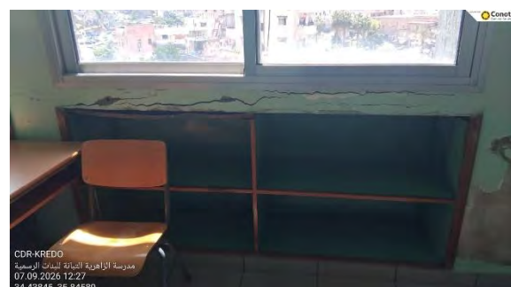
Figure 8 – Crack in Wall
