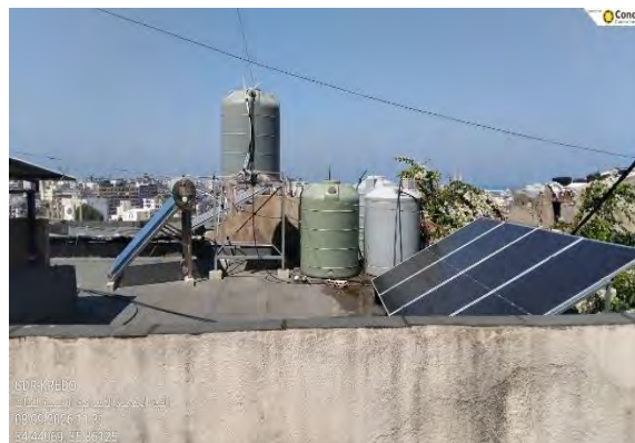
Figure 11- Roof Water tanks leaking
