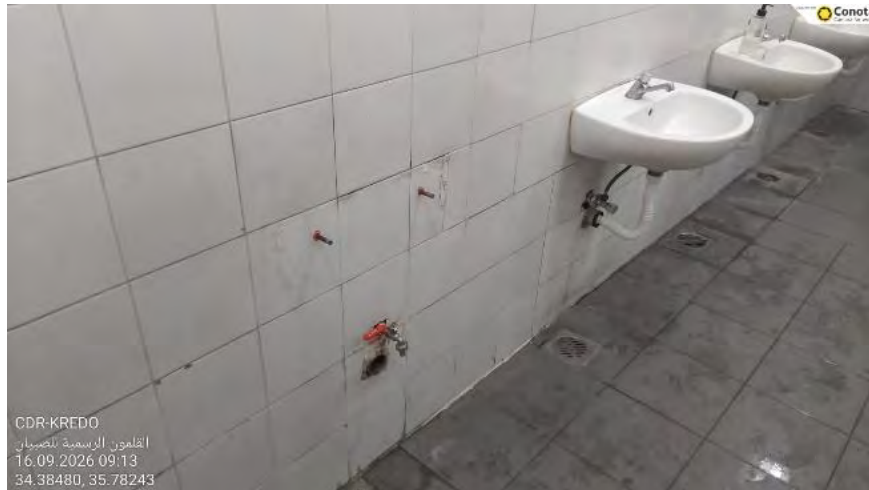
Figure 21 - Missing Wash Basin
