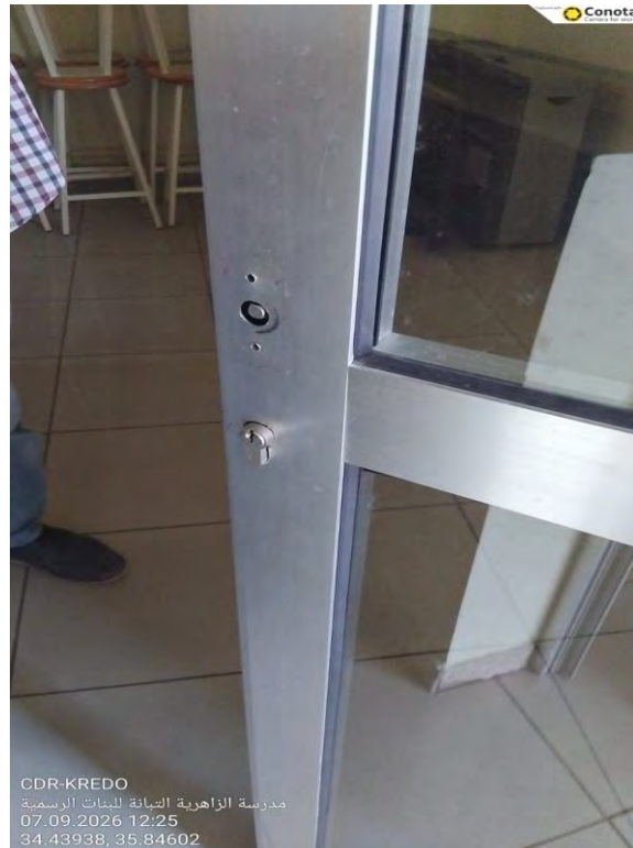
Figure 9 – Missing Door Handle
