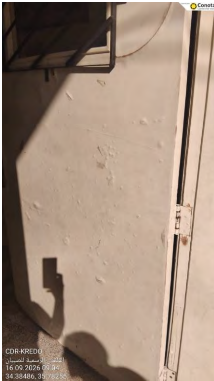
Figure 17 – Damaged Door Paint
