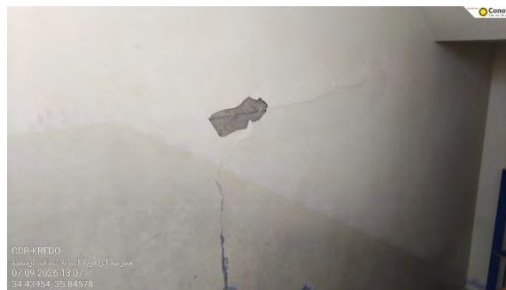
Figure 20 - Crack in Wall
