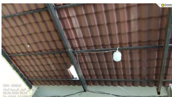
Figure 12 – Broken Playground Cover
