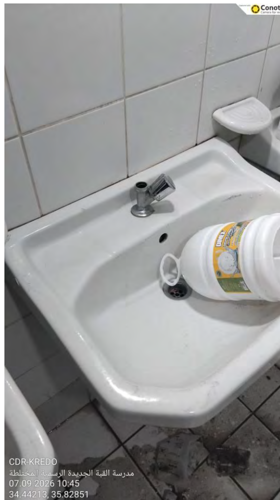
Figure 12 – Missing Wash Basin Accessories
