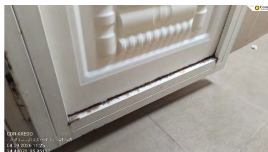
Figure 7- Corrosion and deterioration at the bottom of the steel door
