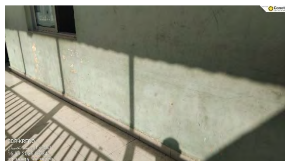
Figure 11 - Damaged Wall Paint
