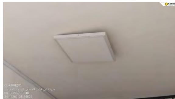
Figure 12 – Damaged Light Fixture
