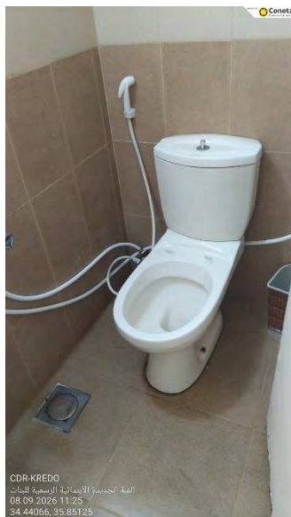
Figure 10- WC cover missing
