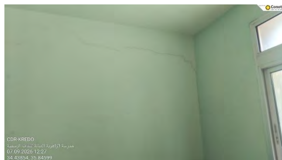
Figure 11 – Crack in Wall
