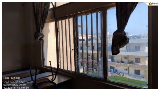
Figure 14 - Broken Window Glass
