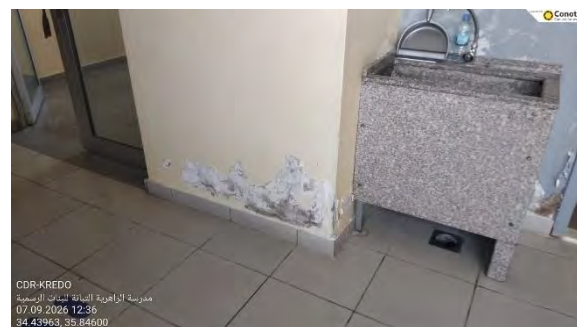
Figure 12 – Humidity in Wall
