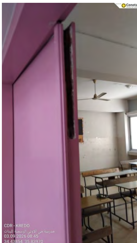
Figure 8 – Missing Door Accessories
