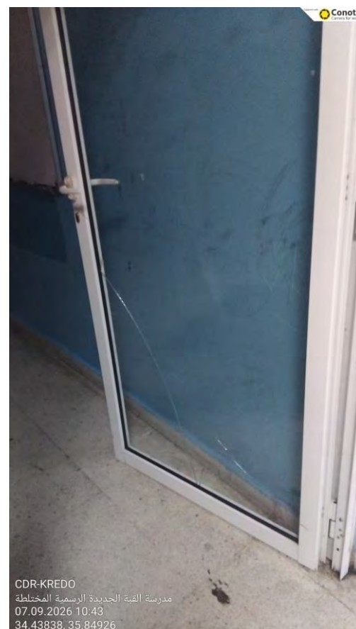
Figure 10 – Broken Door Glazing
