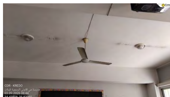
Figure 13 – Damaged Ceiling Paint
