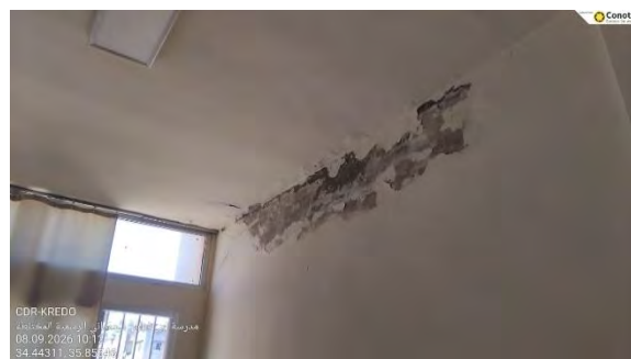
Figure 14 – Humidity in Walls
