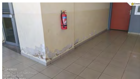
Figure 7 – Humidity in Wall
