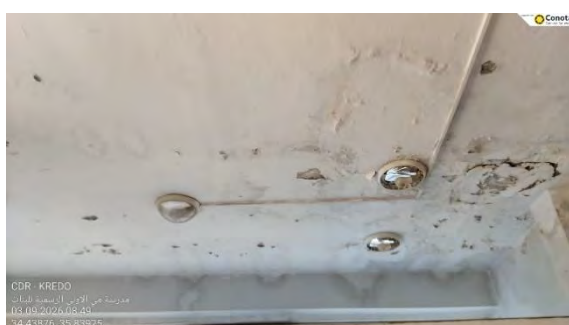
Figure 10 – Humidity in Ceiling
