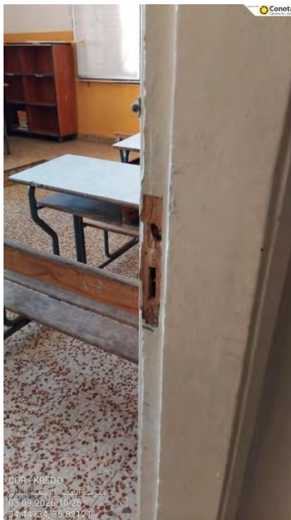
Figure 10 – Missing Door Accessories
