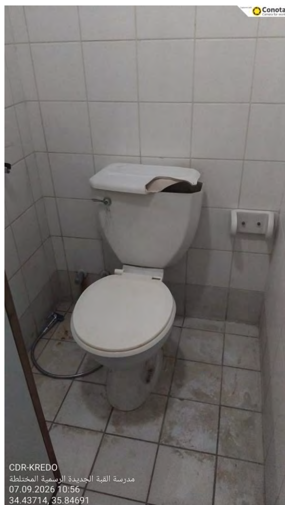
Figure 17 - Broken Toilet Seat
