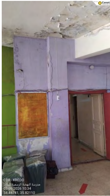
Figure 8 – Column Crack in Playground
