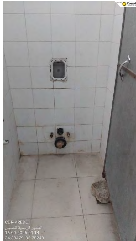
Figure 18 – Missing Toilet Seat
