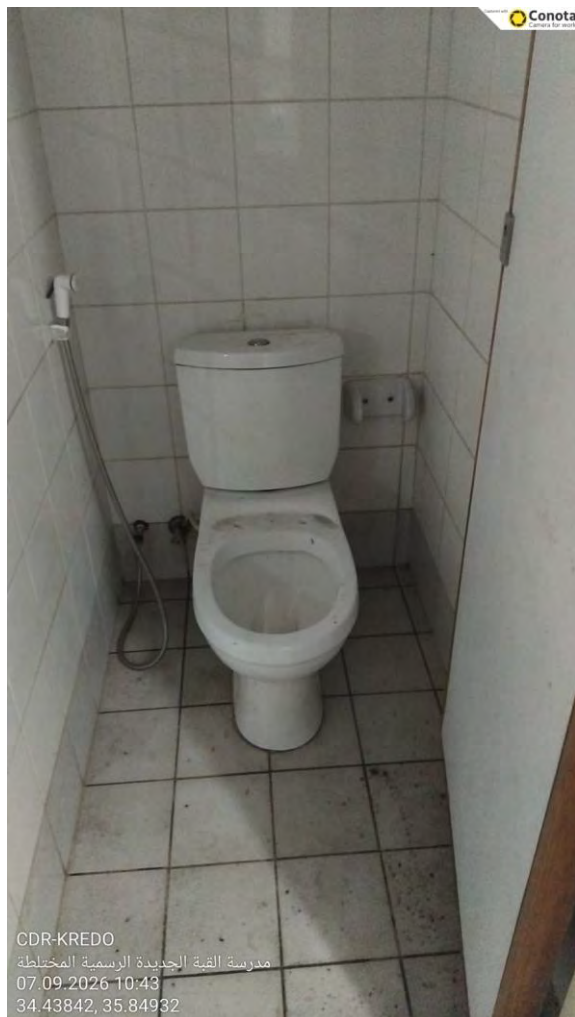
Figure 11 – Missing Toilet Seat Cover
