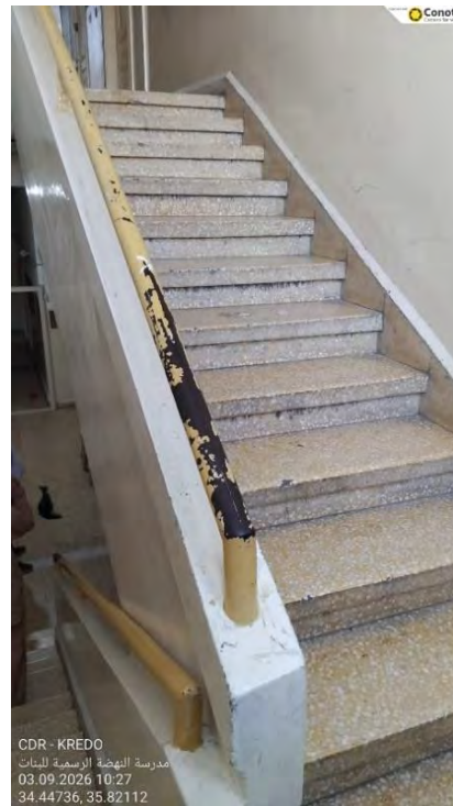
Figure 11 - Damaged Handrail Paint
