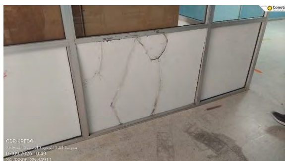
Figure 13 – Broken Partition Panel
