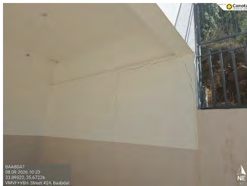
Figure 4 - Humidity in walls
