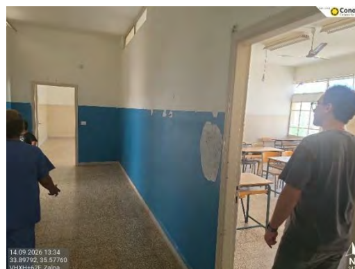
Figure 9- Damaged walls paints
