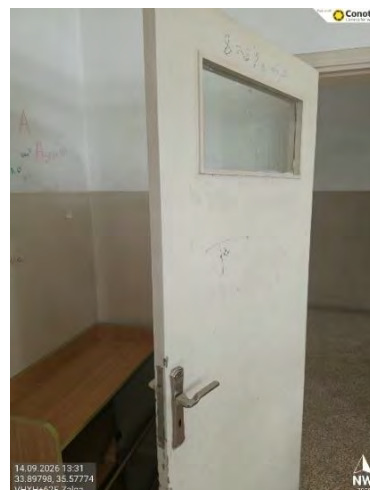
Figure 11- Damaged door accessories
