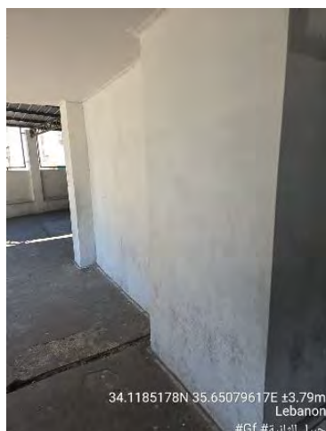
Figure 6- Dirty playground walls
