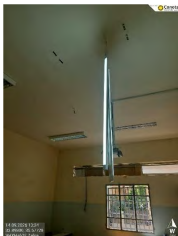
Figure 12- Broken lamps support
