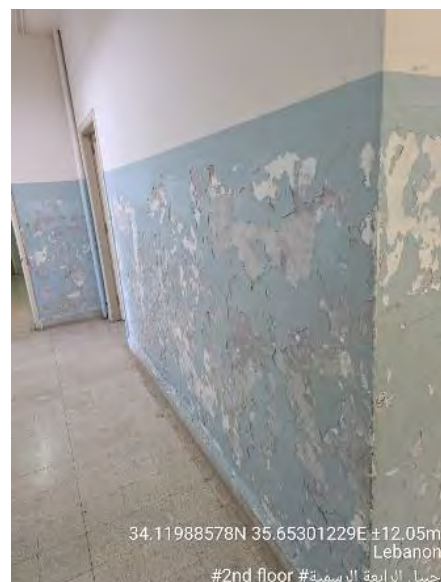
Figure 10- Walls in bad conditions
