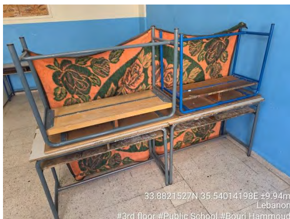
Figure 8- Damaged wall paint
