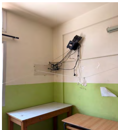
Figure 13- Electrical Reservation Damaged
