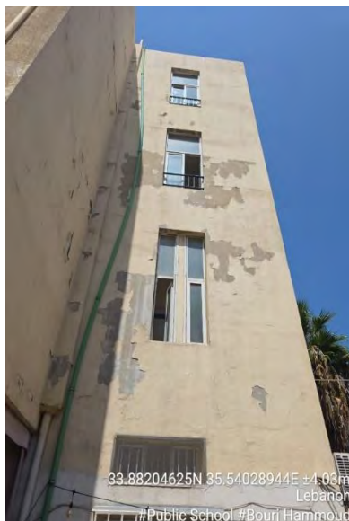
Figure 6- Façade in bad condition
