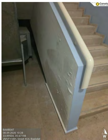
Figure 16 - Damaged staircase paint
