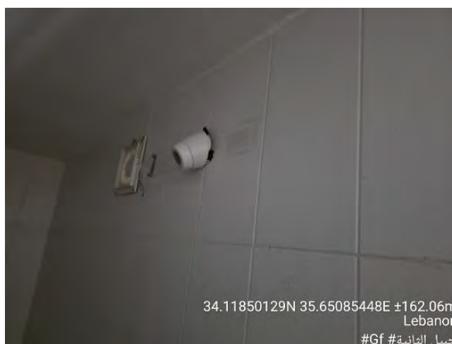
Figure 10- Broken light fixtures
