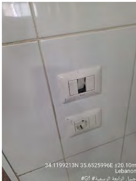
Figure 7- Damaged Switches and Socket
