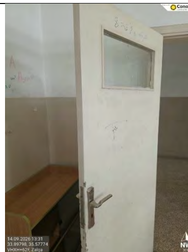
Figure 11- Damaged door accessories
