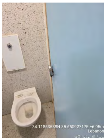
Figure 8 - Damaged door handle
