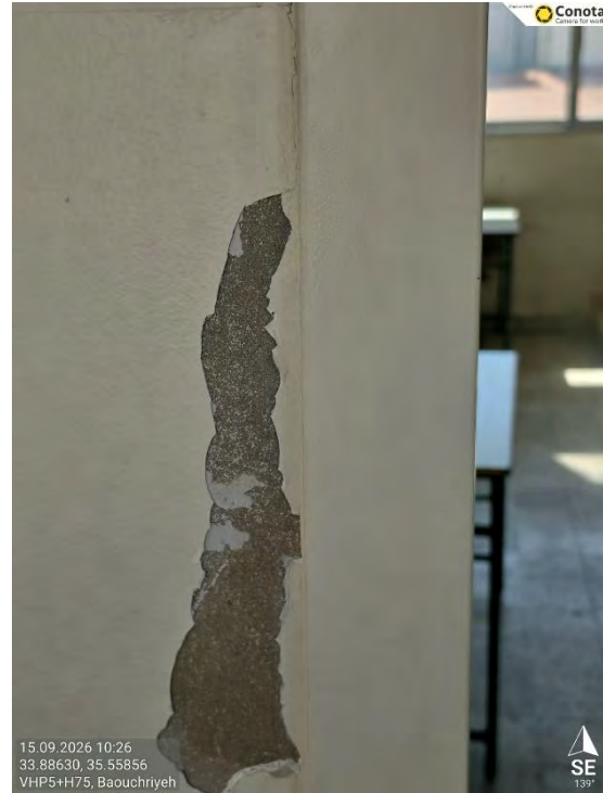
Figure 9 - Damaged wall paint
