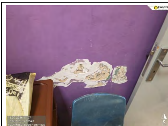
Figure 4 – Damaged wall plastering
