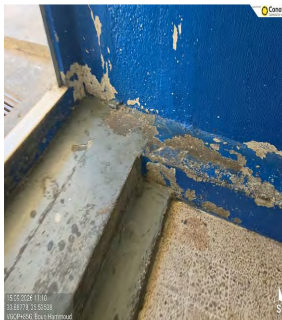
Figure 11- Wall stairs in bad condition
