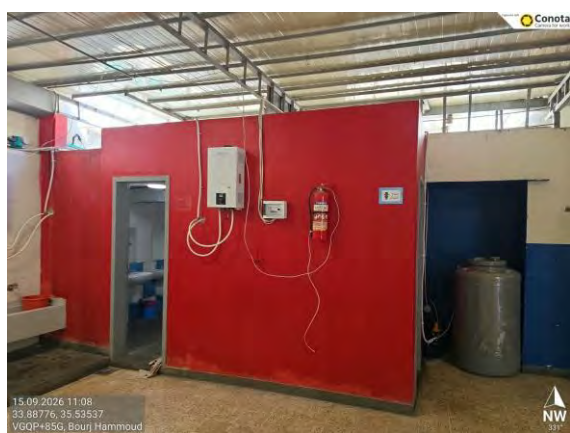
Figure 7 - Electrical cables in bad condition
