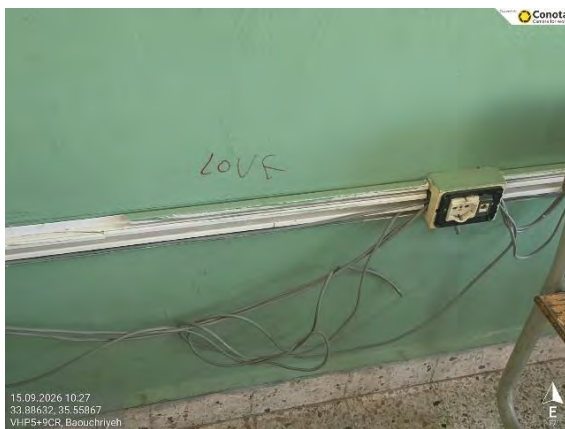
Figure 10 - Damaged electrical routing
