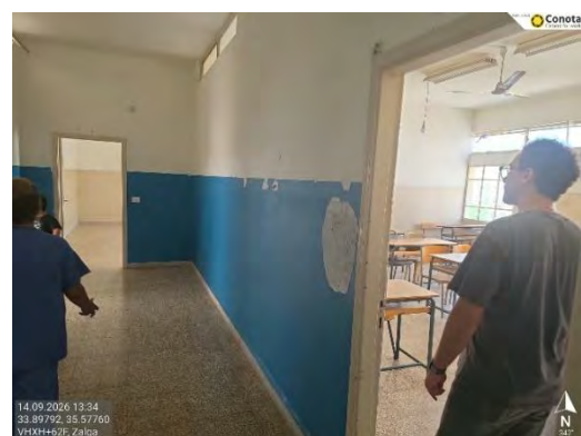
Figure 9- Damaged walls paints
