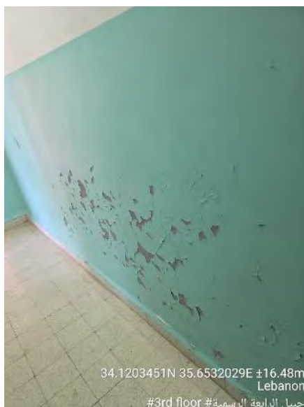
Figure 9- Walls in bad conditions
