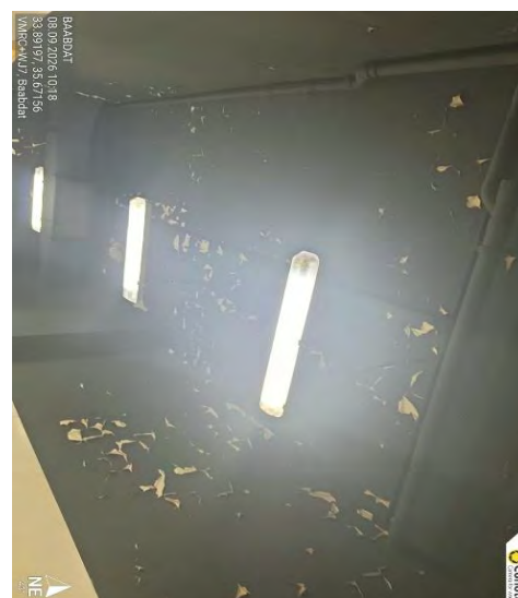
Figure 9 - Damaged roof paint
