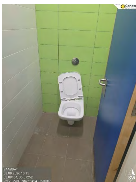
Figure 14 - Damaged toilet accessories
