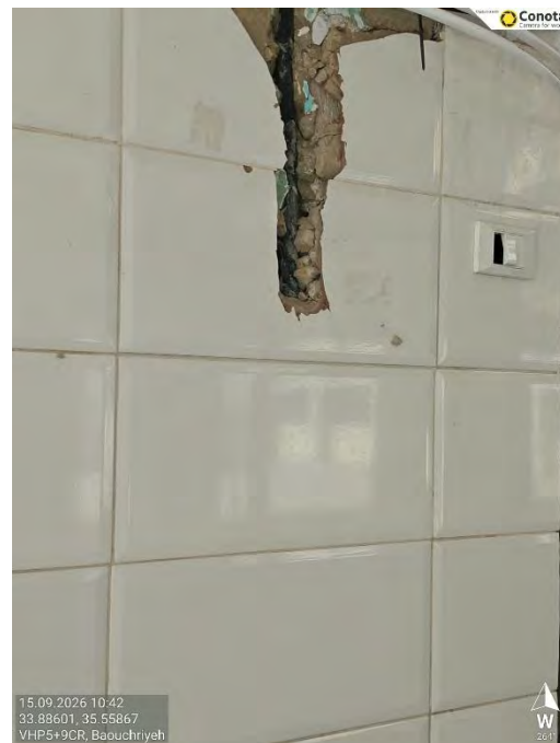
Figure 7 - Damaged wall tiles
