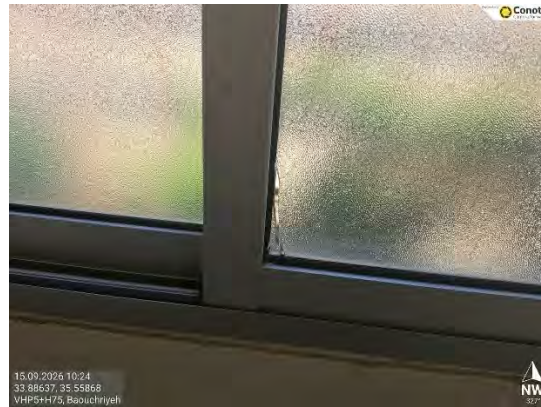
Figure 5 - Damaged Aluminum Glazing
