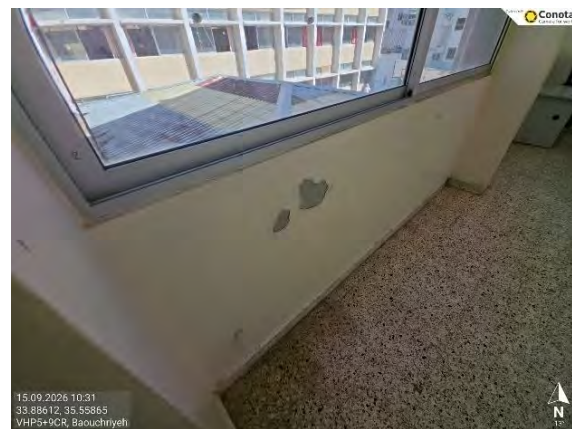
Figure 11 - Damaged wall paint
