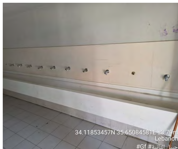
Figure 9 - Water taps not available
